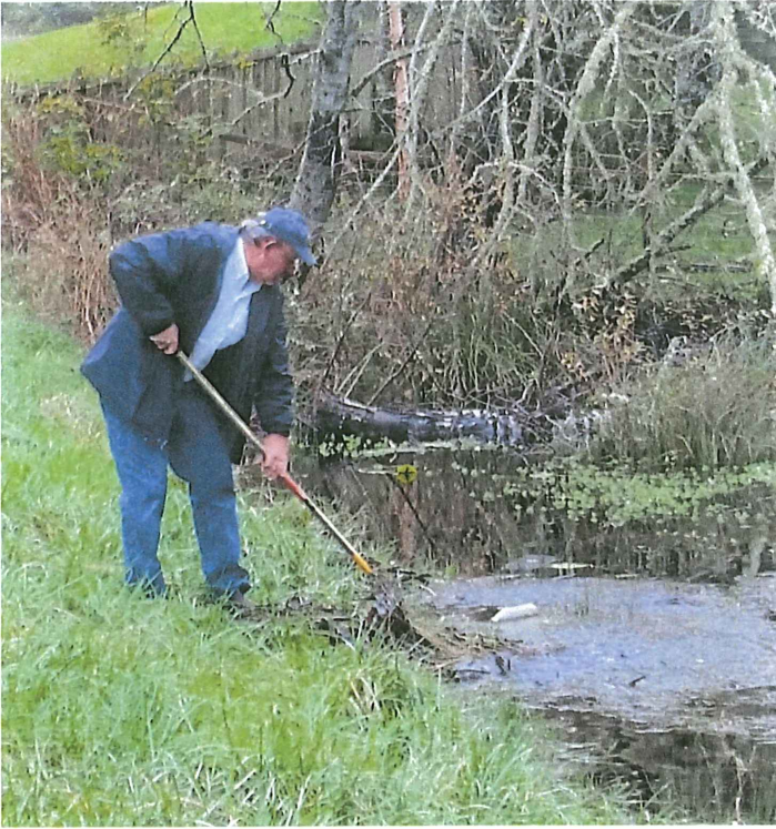
Smith Lake Residents Clearing 9 th Street Culvert Obstructions (left) and Clearing Debris from the Cemetery Weir (right)
