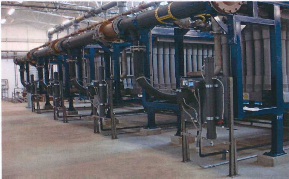
Multiple turbidity units on CMF Train 1
