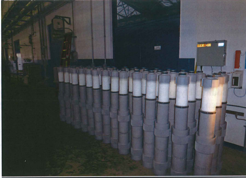
New Filters ready to be installed Dec 2012
