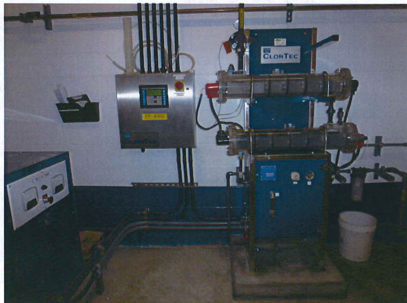
Sodium Hypochlorite Generation system
