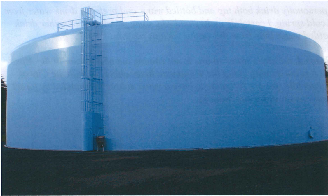
3.5 Steel Reservoir at Water Facility
