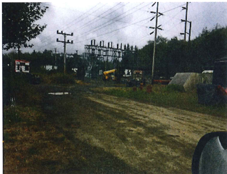
Power Substation at South End of SE Jetty
