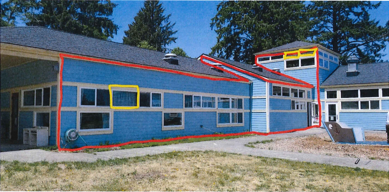
East Wall South Wing (Failed windows in yellow)
