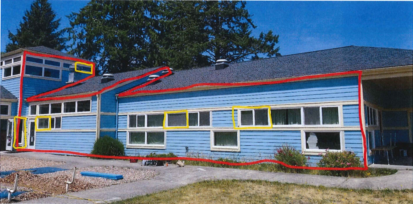
South Wall East Wing (Failed windows in yellow)
