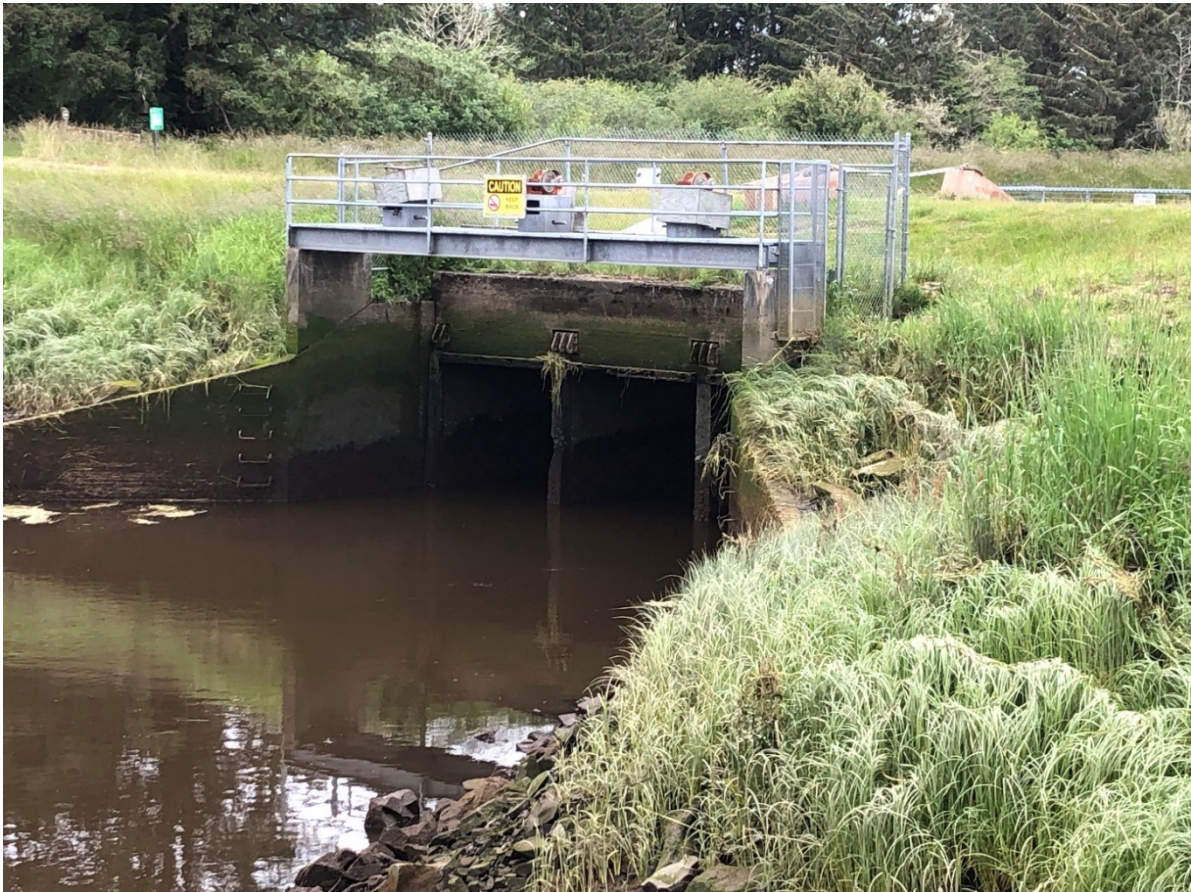
Photo: 8 th Street Dam and Culverts Looking Upstream (Location of the Former Tidegates).
