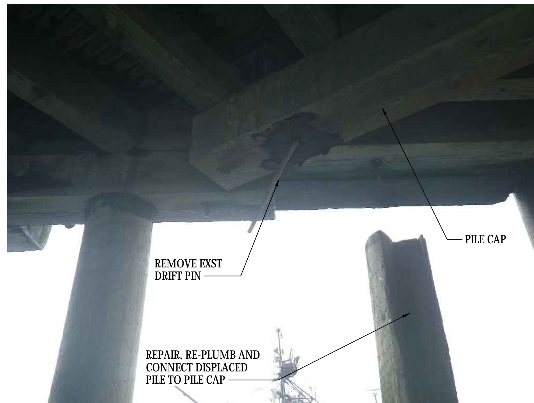
11 PHOTO - DISPLACED PILE AT WP31/D S-10 SCALE: NTS
