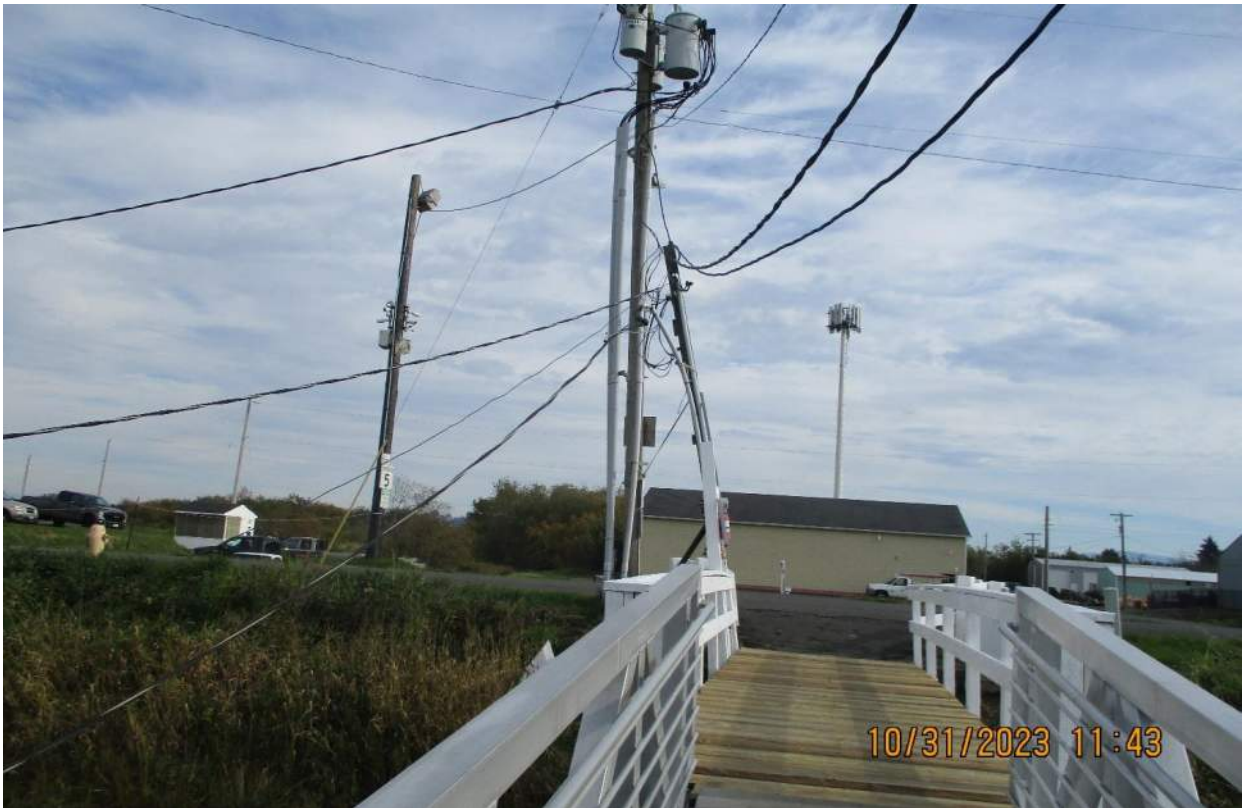
Photo 16: Handrail being pulled down by utility pole.
