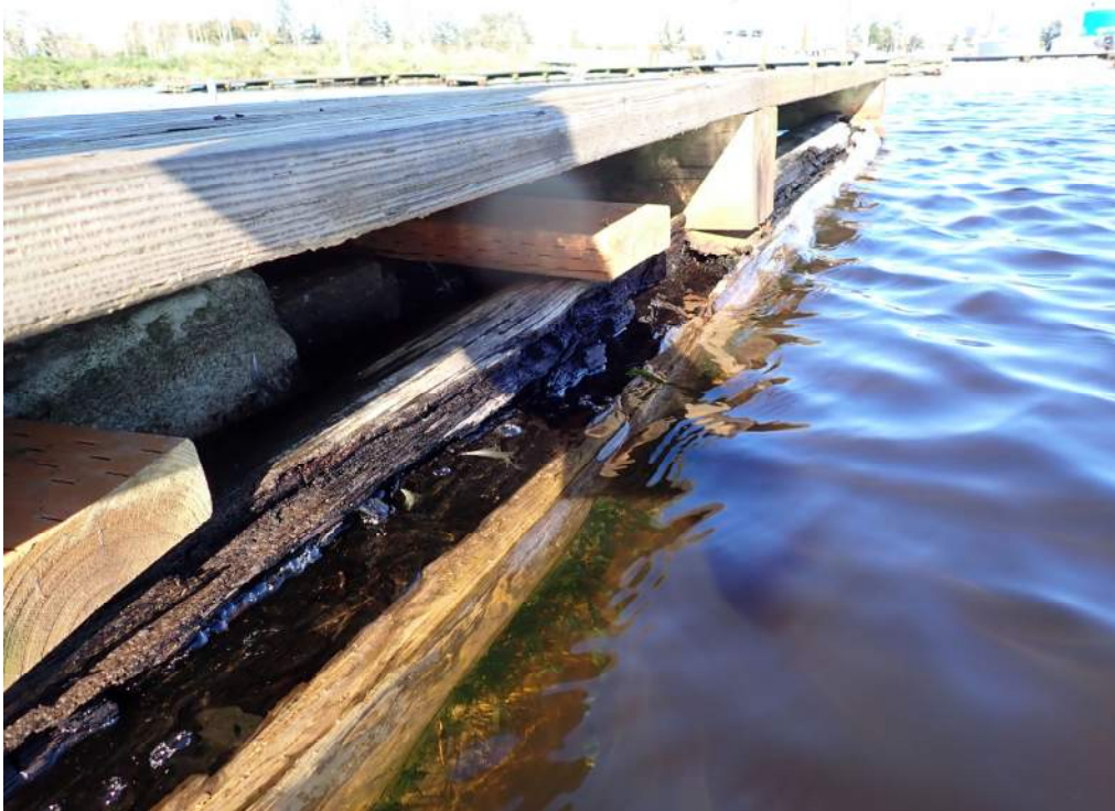
Photograph 20– Typical Area of Severe Section Loss in Timber Floats
