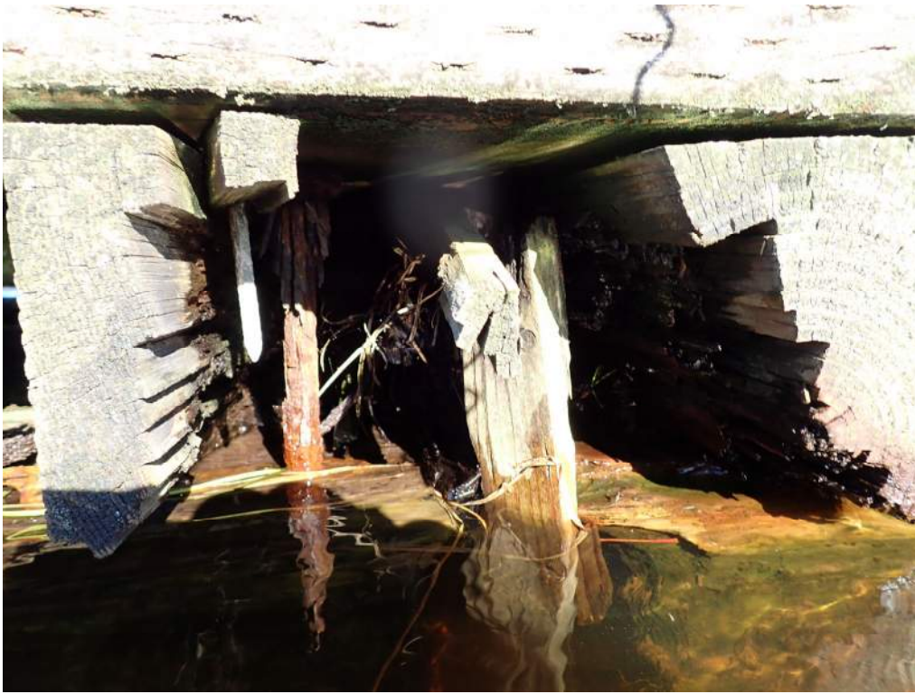
Photograph 29– Loose Connection Between Timber Float and Transverse Timber Support
