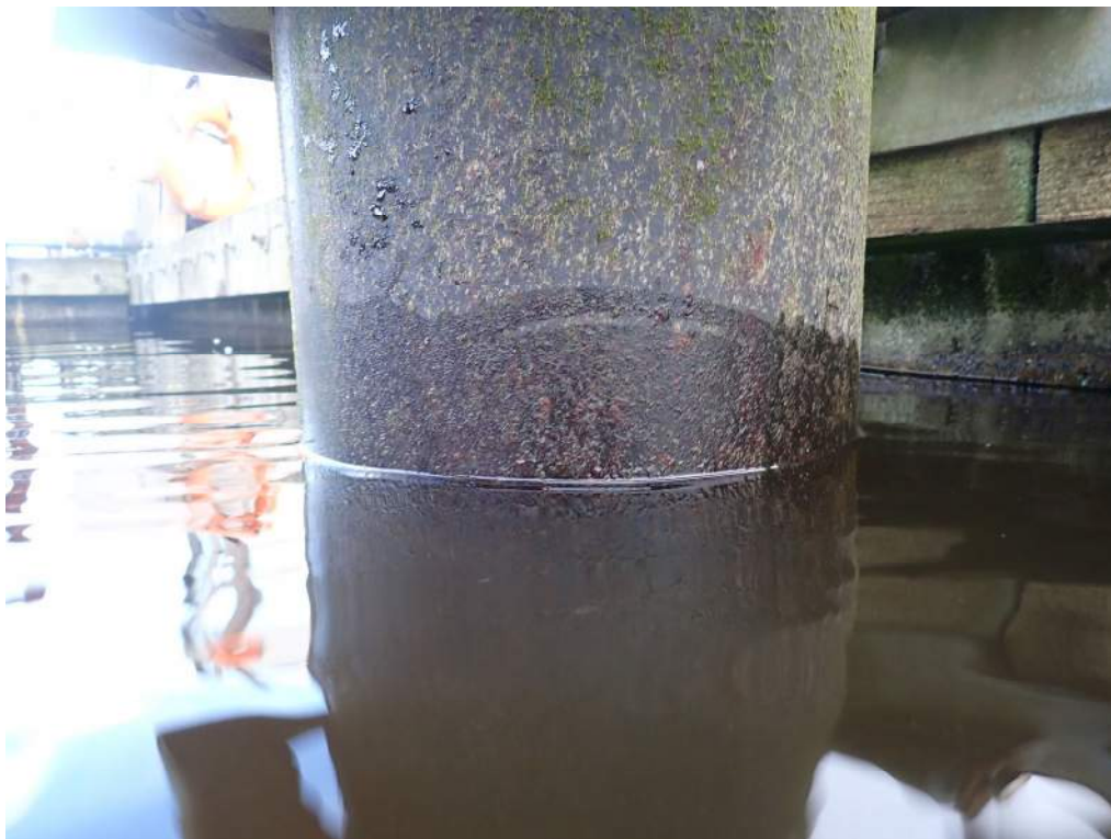
Photograph 12– Typical Steel Guide Pile at Waterline
