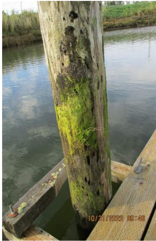
Photo 1: Typical condition of timber piling. Note marine growth near the waterline.
