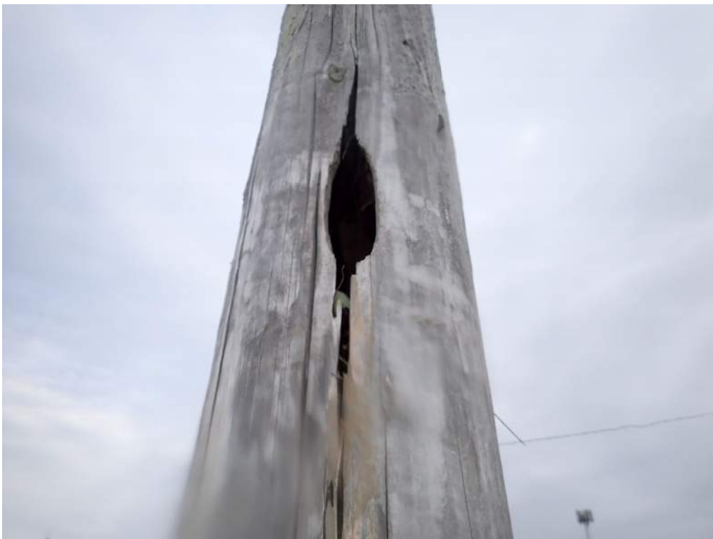
Photograph 26– Typical Severe Loss of Section in Timber Guide Piles
