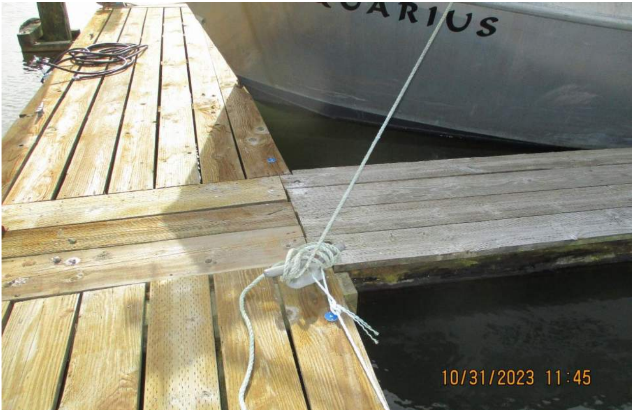
Photo 28: Ledge type connection where finger pier meets main walkway.
