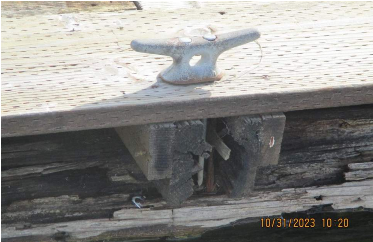
Photo 24: Typical condition of cleat. Cleat is only restrained by the deck, stringer below is decayed.
