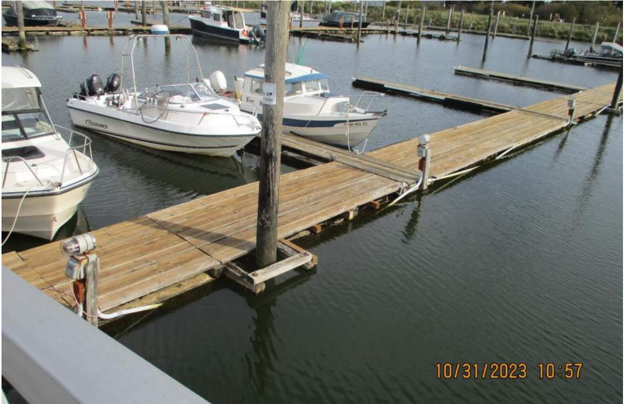
Photo 4: Typical wooden pile hoop.
