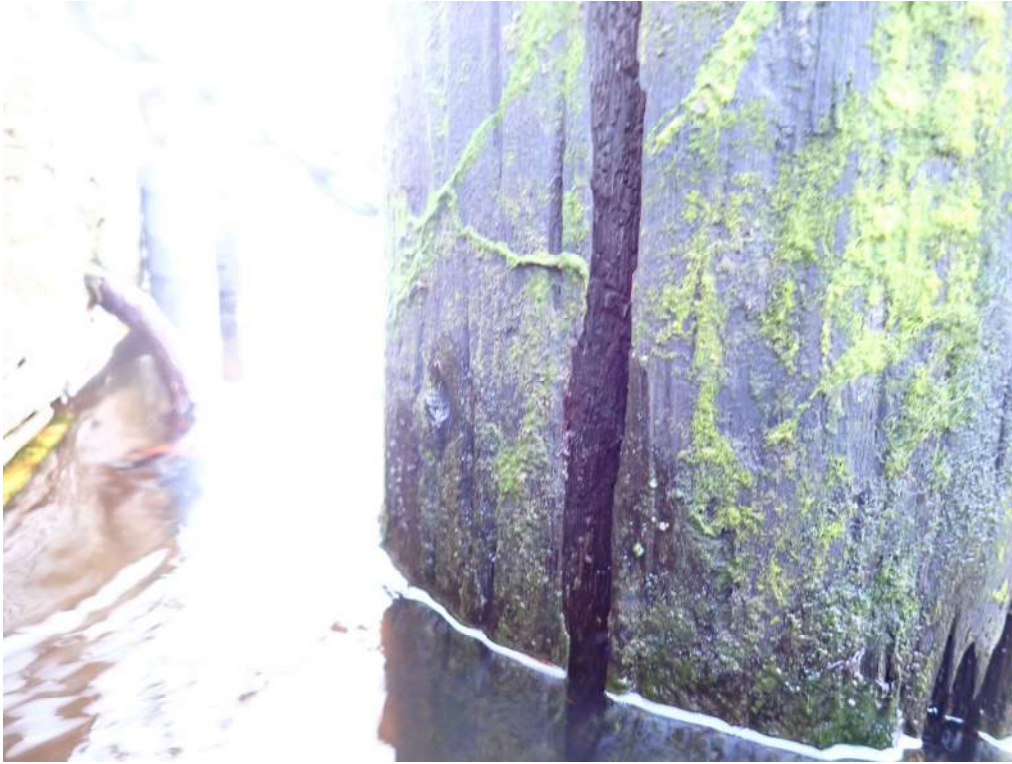
Photograph 27– Typical Check in Timber Piles
