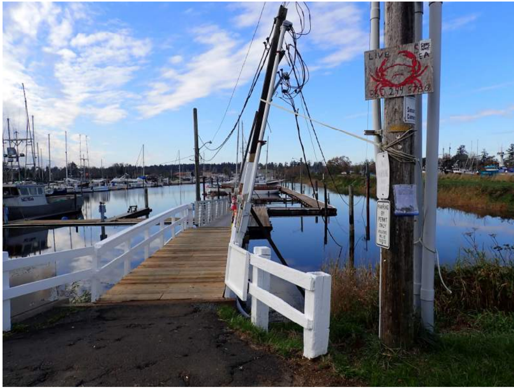
Photograph 17– Unstable Utility Line Post at Northeast Marina Entrance Looking West
