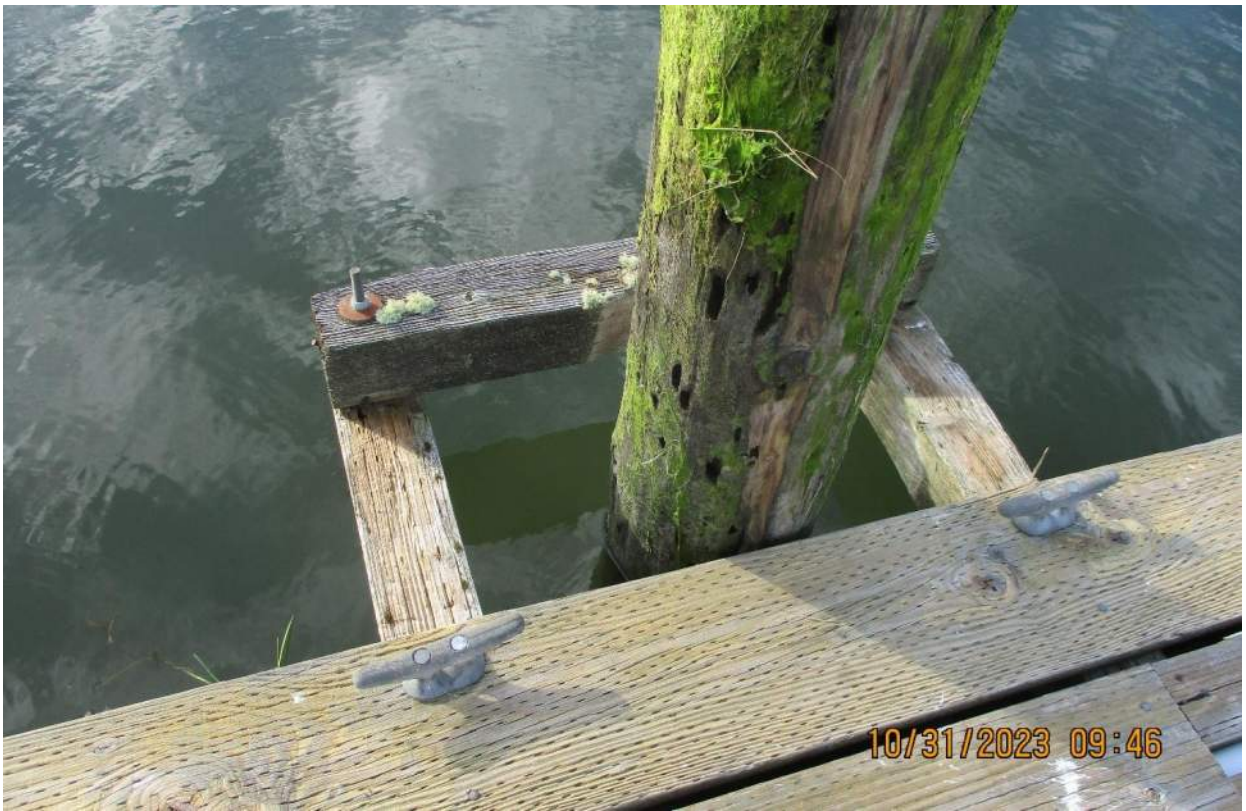
Photo 2: Close up showing possible marine borer activity.
