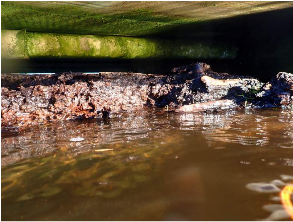
Photograph 19– Typical Area of Severe Section Loss in Timber Floats
