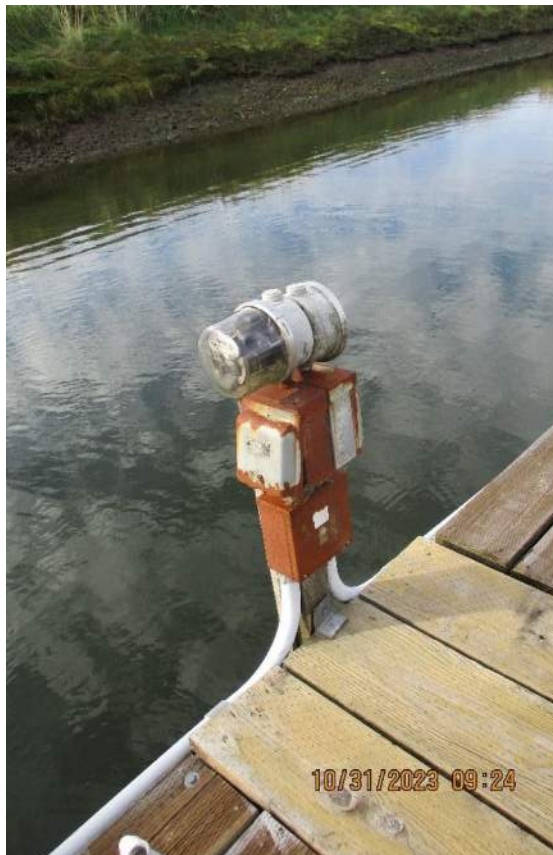
Photo 22: Typical utility pedestal.
