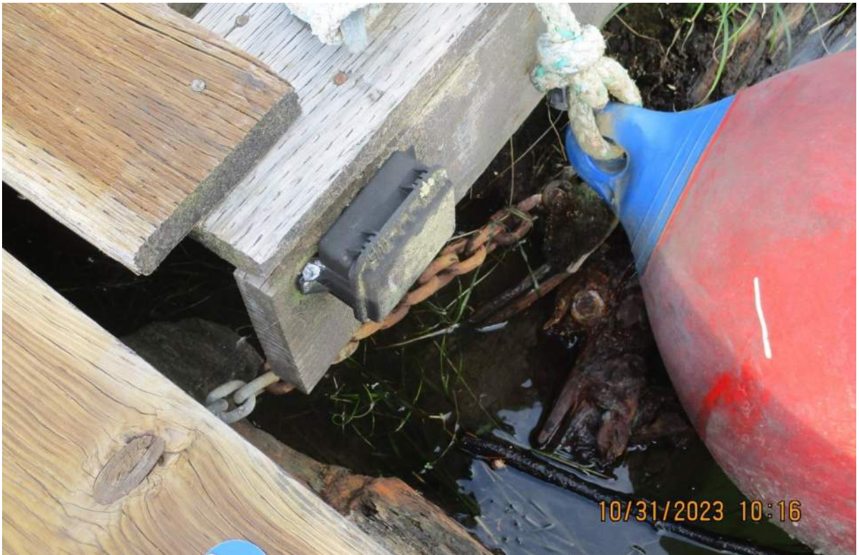
Photo 26: Decayed chain connect. Note corrosion in chain and heavily corroded hardware in float log.
