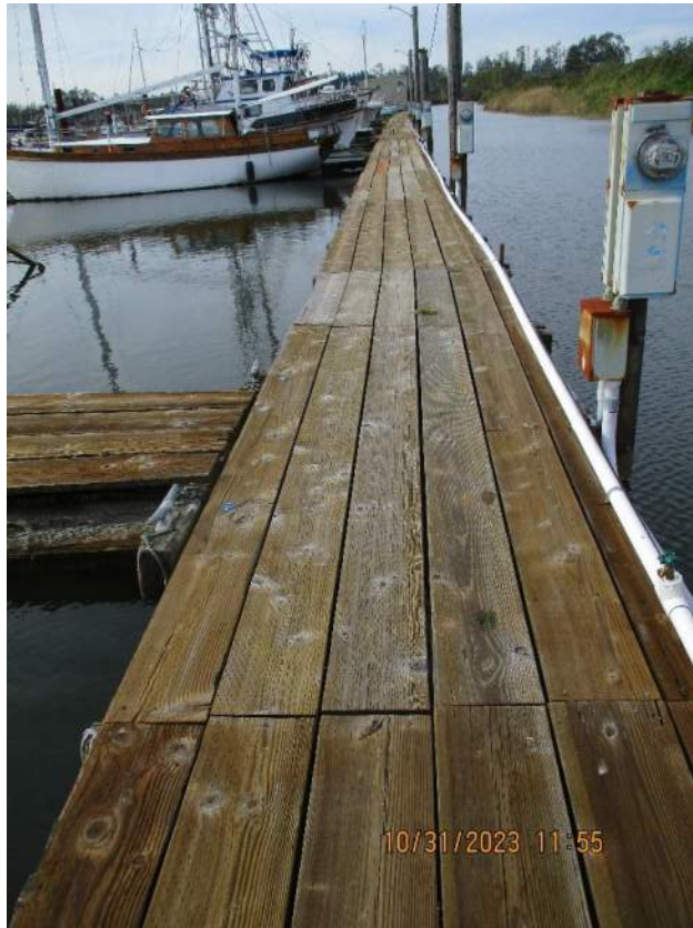
Photo 23: Recently replaced water piping along Dock N. Should be a model for future piping repairs.
