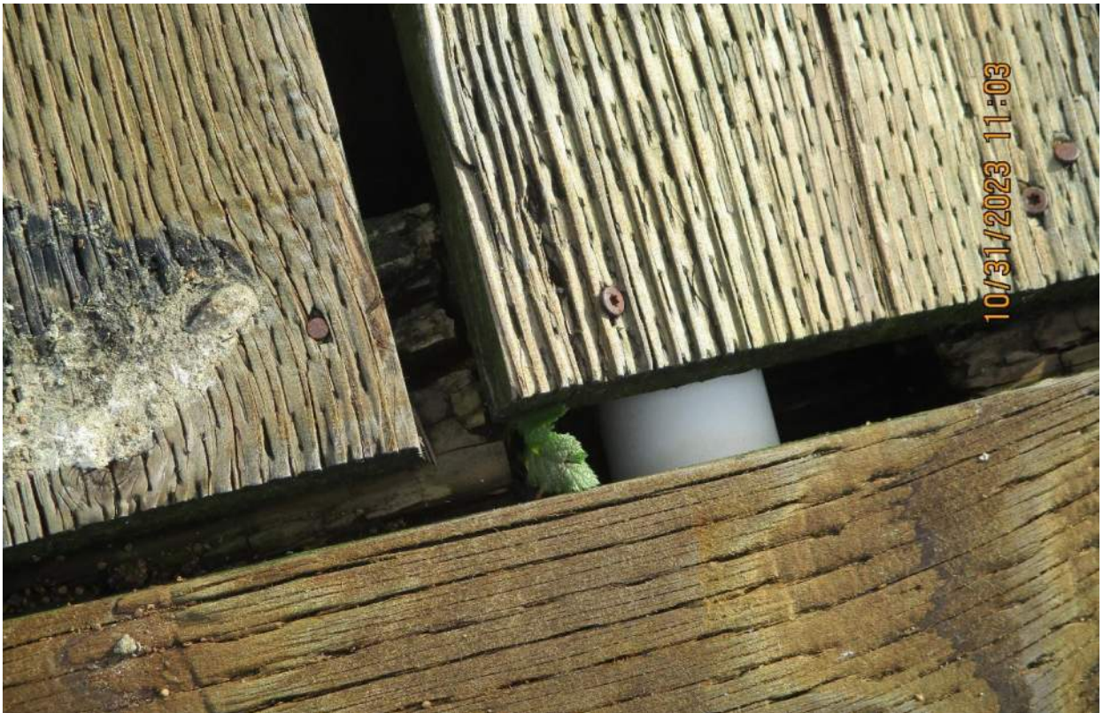
Photo 14: Example of cut stringer to allow for water pipe to be installed below the deck.
