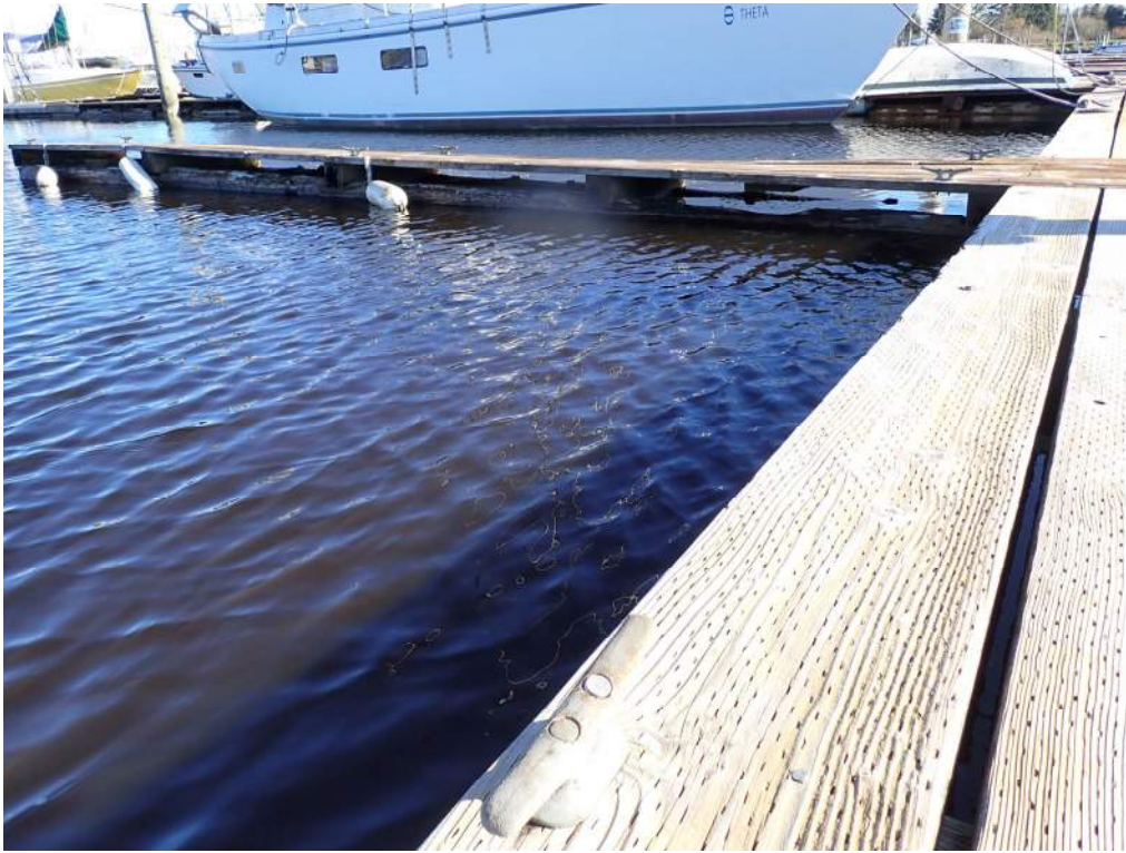
Photograph 31– Typical Rotated Finger Pier (Dock C, between Slips 65 and 66)
