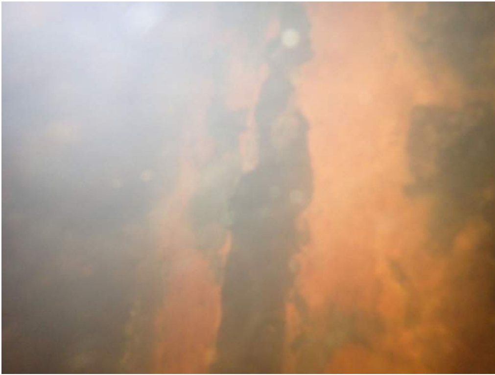
Photograph 23– Corrosion Hole in Steel Pile at Dock A , Between Slips 27 and 28
