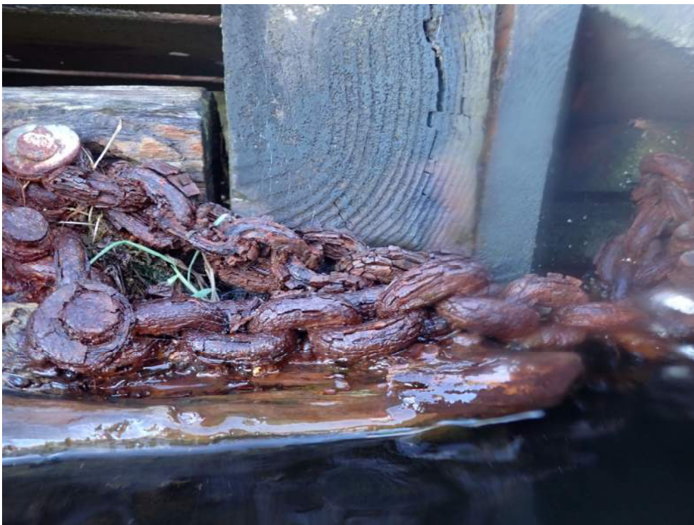
Photograph 30– Flaking Rust at Chain Connection at Dock C, Slip 36
