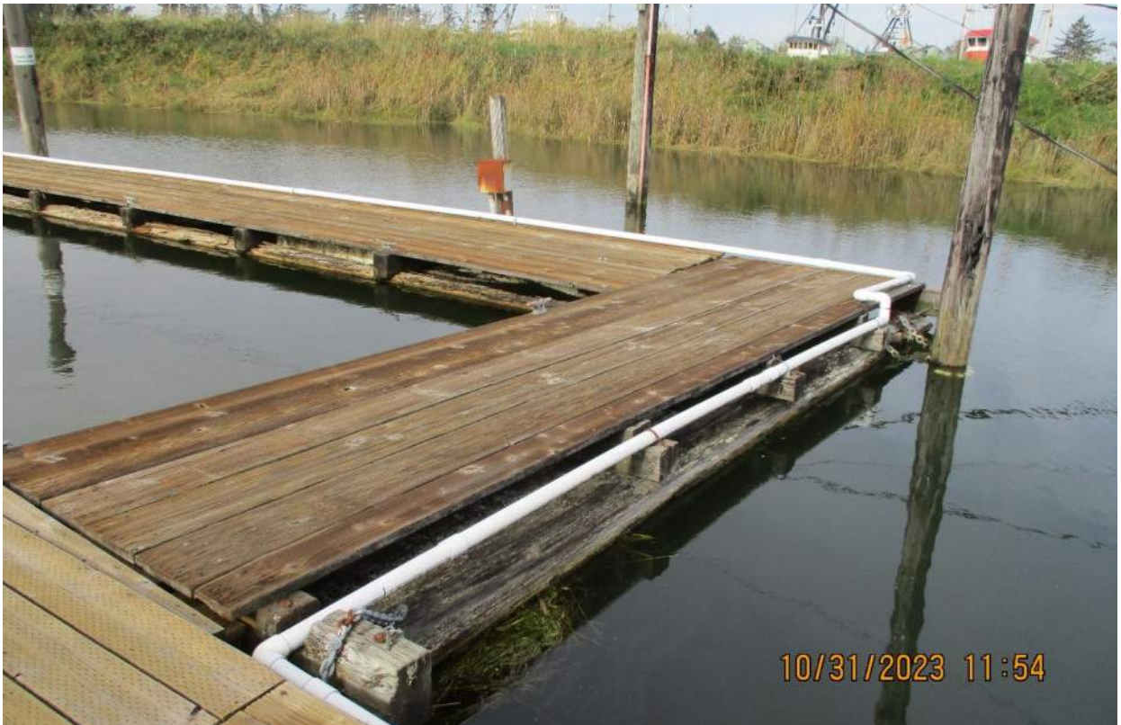
Photo 8: Corner where Dock M and N meet. Note the sag in the corner due to lack of float log buoyancy.
