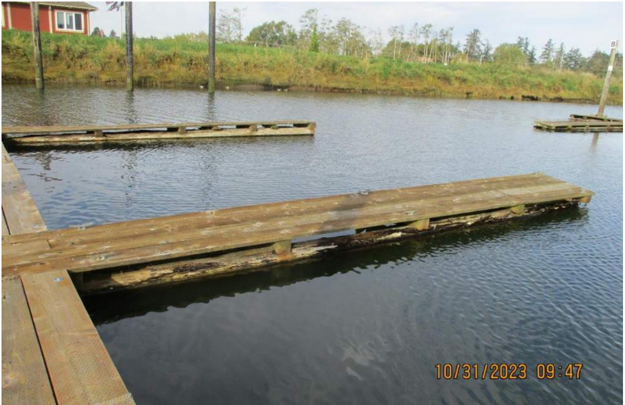
Photo 7: Uneven finger piers due to lack of buoyancy in float logs.
