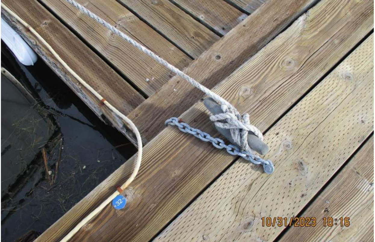
Photo 25: Chain connection, with lag bolt into the deck. Unclear if lag bolt is into stringer below.
