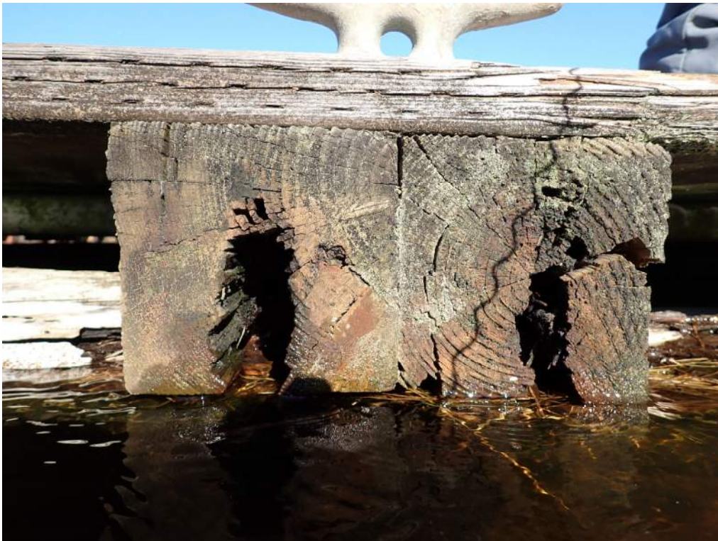
Photograph 28– Typical Section Loss in Timber Transverse Supports
