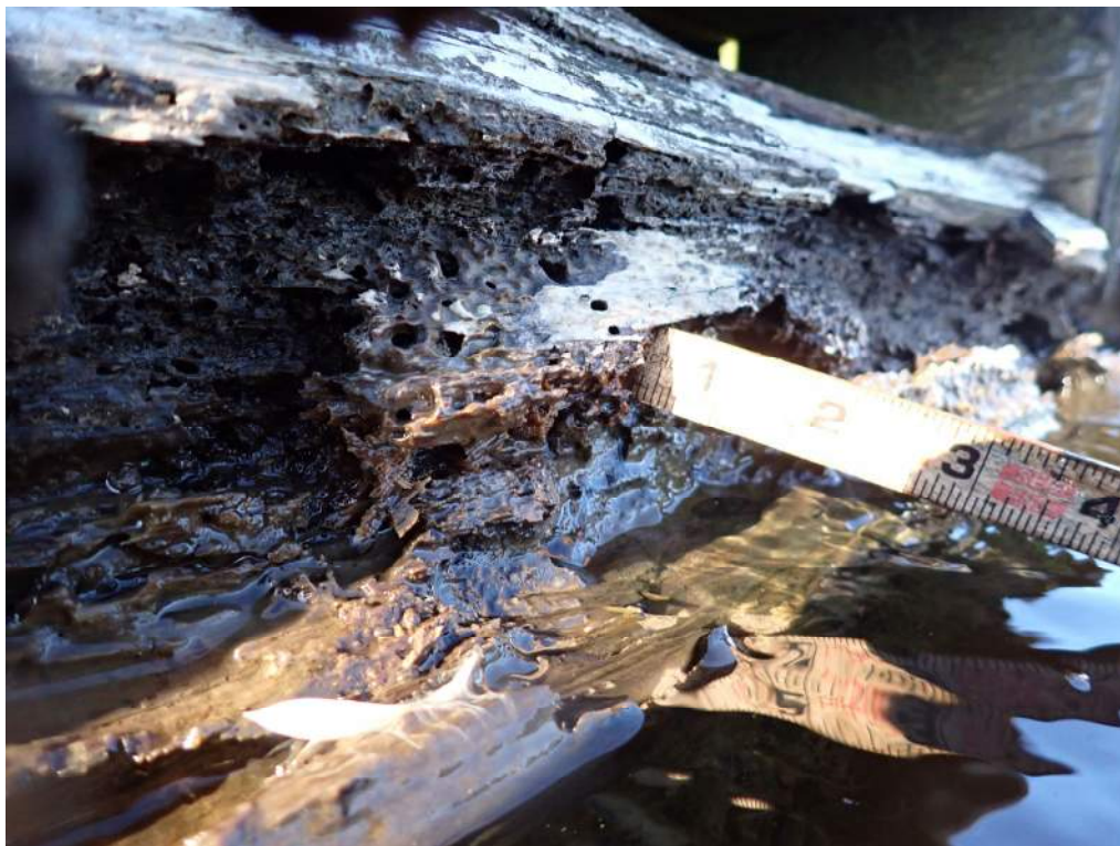
Photograph 18– Typical Evidence of Marine Borers in Timber Floats
