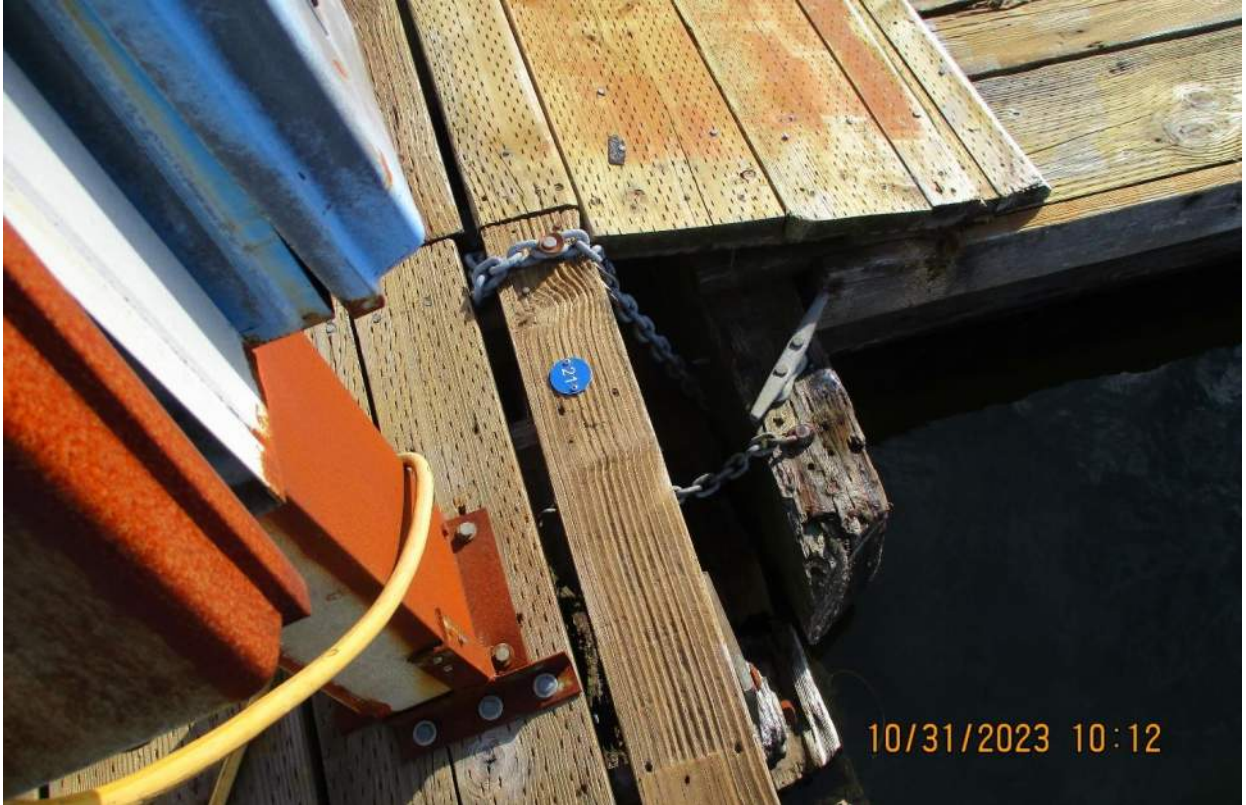
Photo 27: Chain connection, lagged into deck only.
