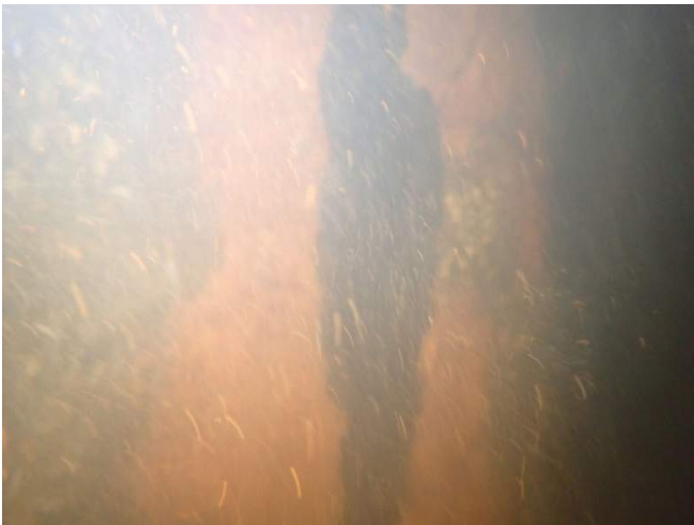
Photograph 24– Corrosion Hole in Steel Pile at Dock A, Between Slips 25 and 26
