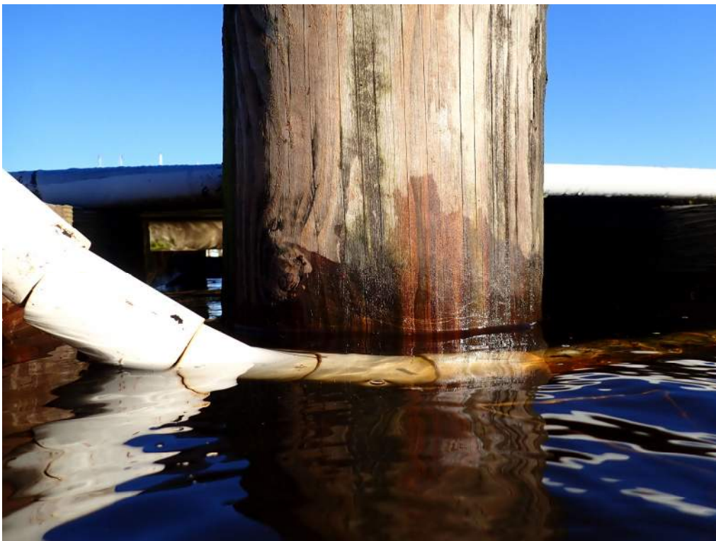
Photograph 10– Typical Timber Guide Pile at Waterline
