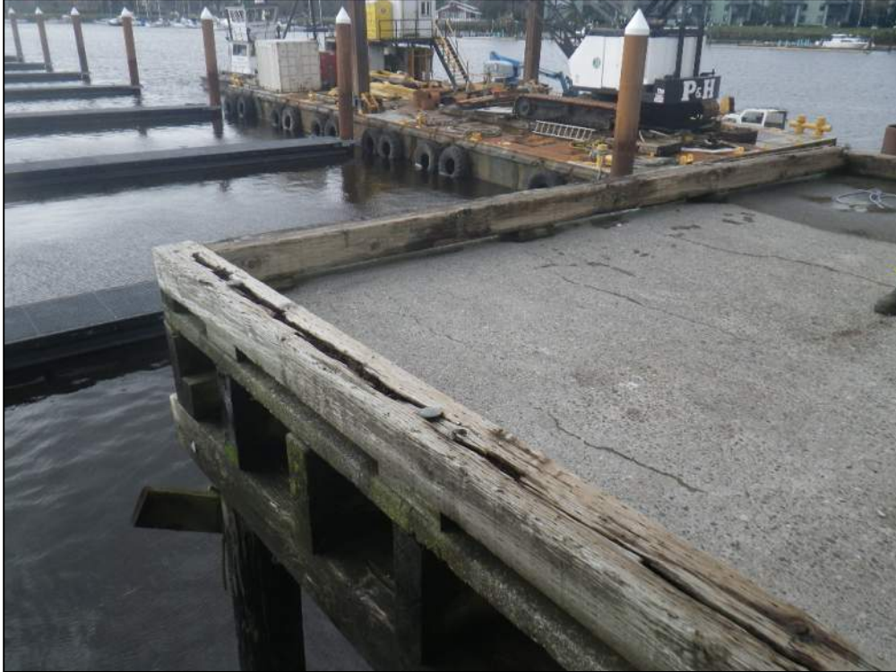
Photo 33. West Trestle Bullrail Decay At Bent WT8
