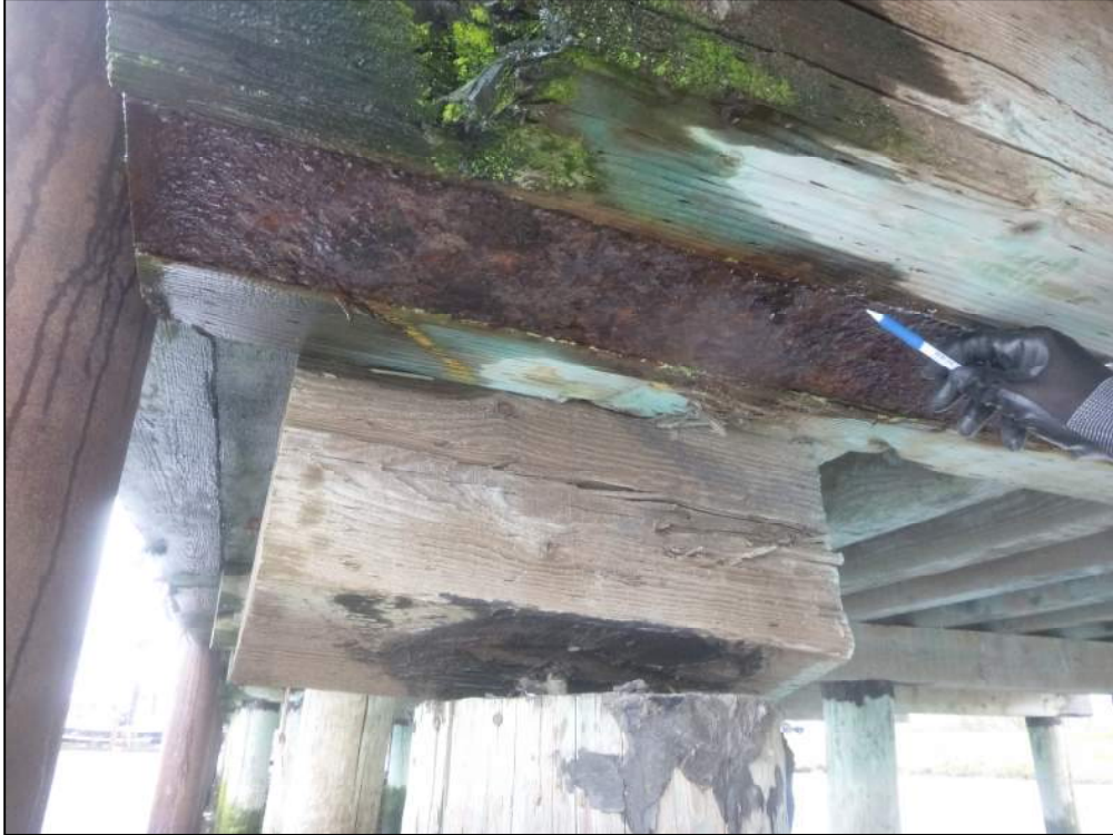
Photo 19. Typical Steel Beam Corrosion (Bent WP13)
