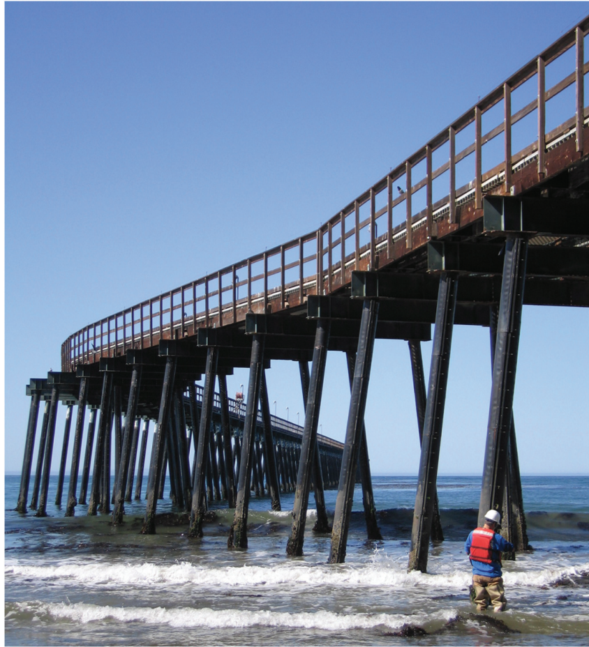
Fig. A-11. Steel ocean pier; note height of deck that cannot be adequately inspected from water or shore
