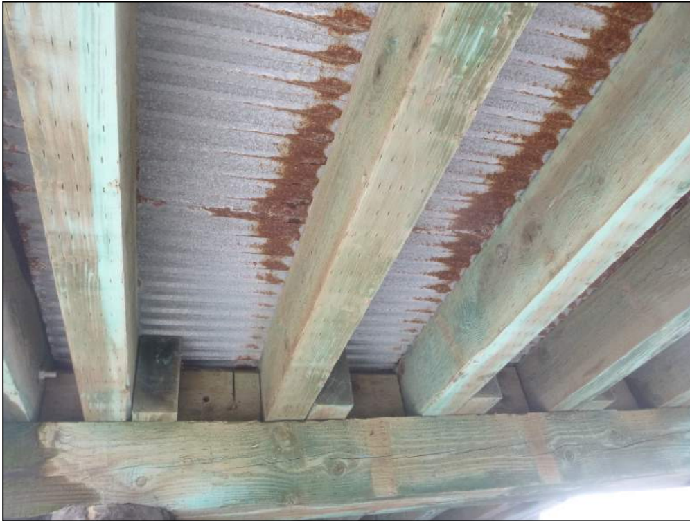
Photo 31. East Trestle Typical Deck Corrosion (Bent ET5)
