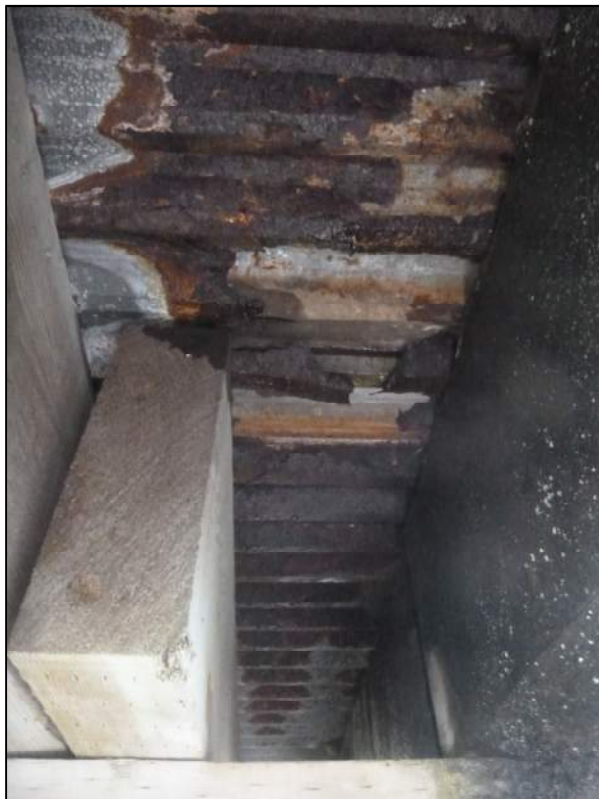
Photo 28. West Trestle Steel Deck Corrosion And Section Loss At Bent WT4
