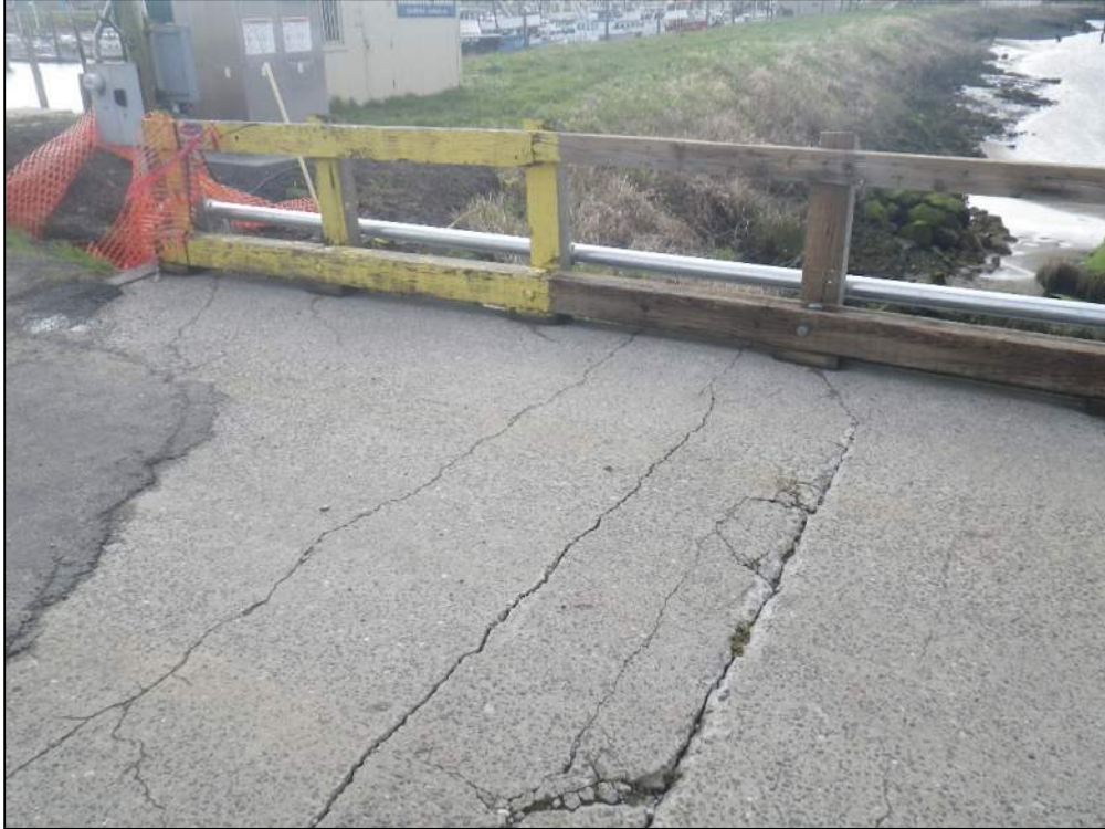
Photo 23. West Trestle Cracks And Spalls Between WT0 And WT2
