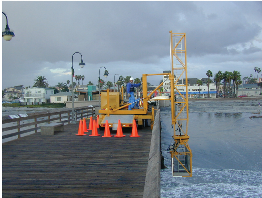
Fig. A-2. Above water inspection team using a man lift to access the underside of a timber pier deck
