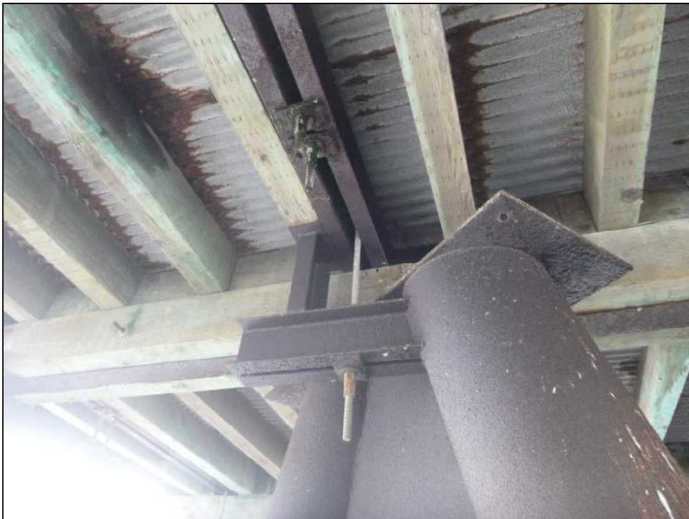
Photo 20. Typical Corrosion At Miscellaneous Steel Beams (Bent WP27)
