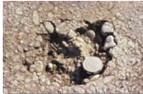
Condition State 2 (CS 2)
