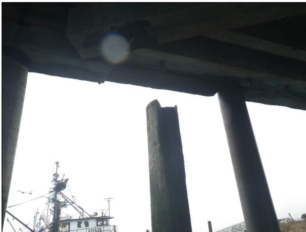
Photo 12. Displaced Pile At WP31/D
