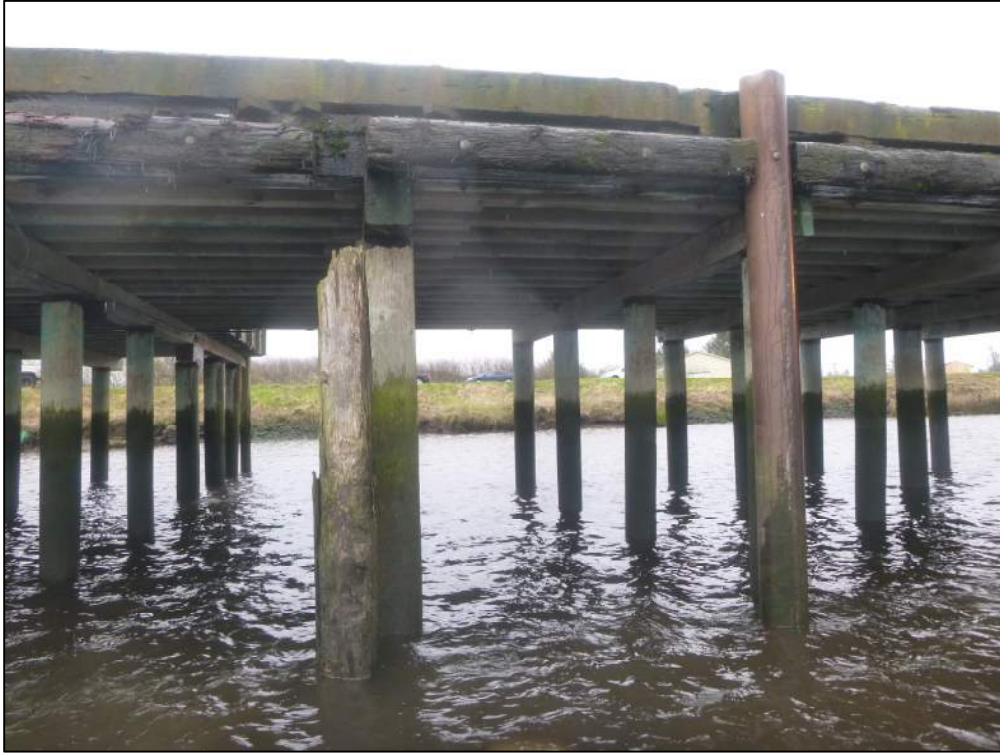
Photo 21. Typical Fender Pile Corrosion And Broken Timber Pile (Bent WP24/25)
