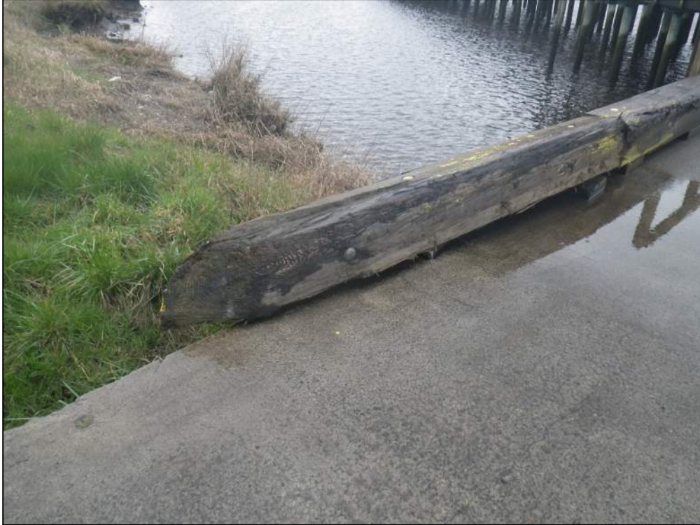
Photo 39. East Trestle Displaced Bullrail (Bent ET0 to ET0.5)
