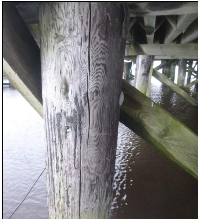
Photo 10. Typical Pile Crack (Pile WT5/C)
