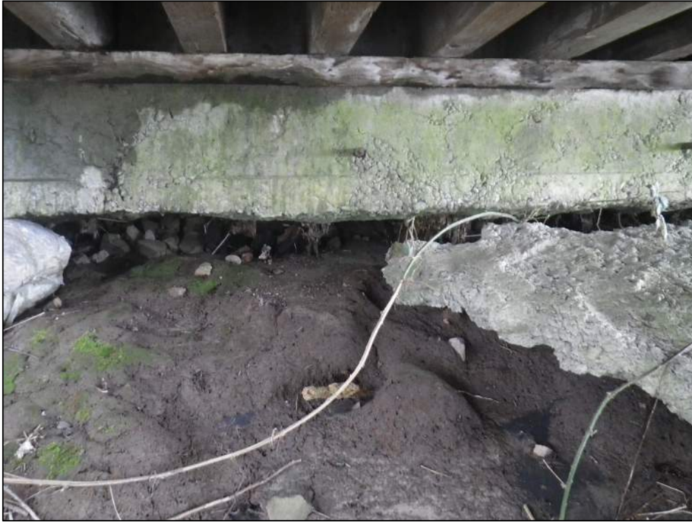
Photo 7. West Trestle Abutment Scour And Timber Pile Decay
