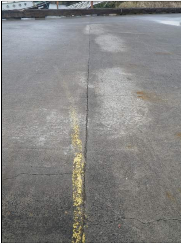
Photo 29. Work Pier Typical Construction Joint And Cracks (Pile Row WPD Looking West)
