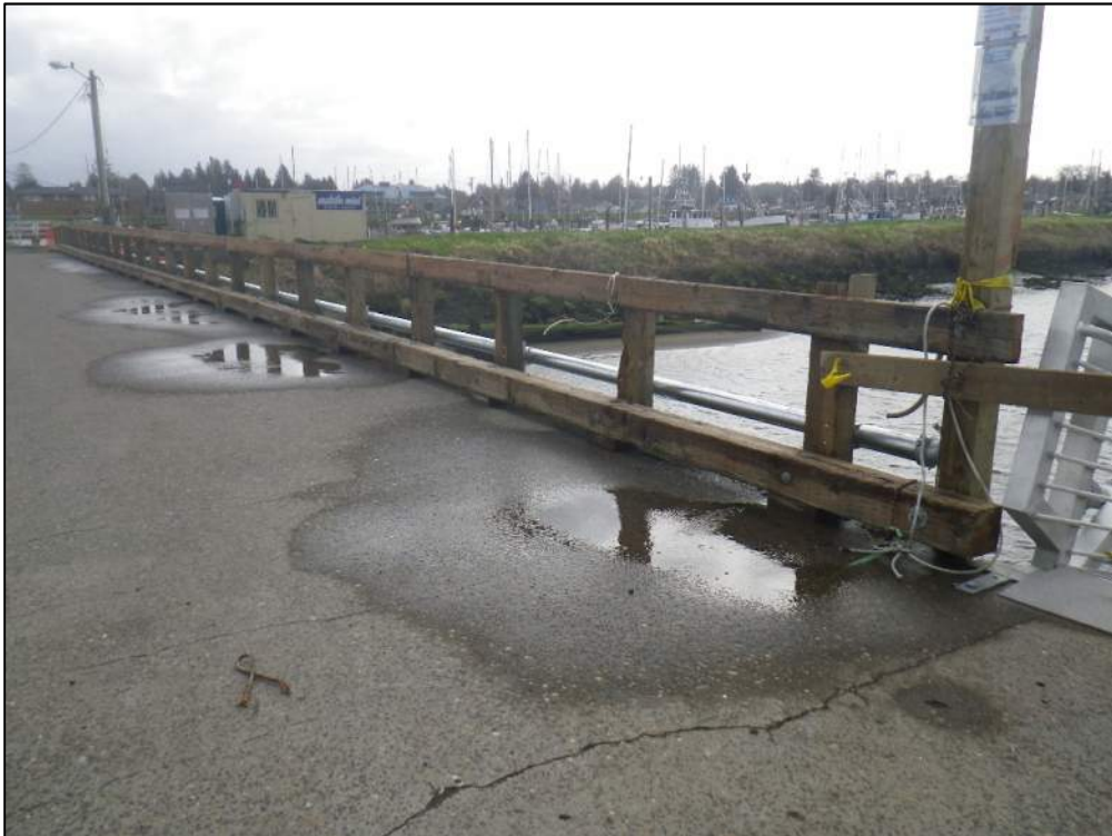
Photo 22. West Trestle Typical Deck Cracks
