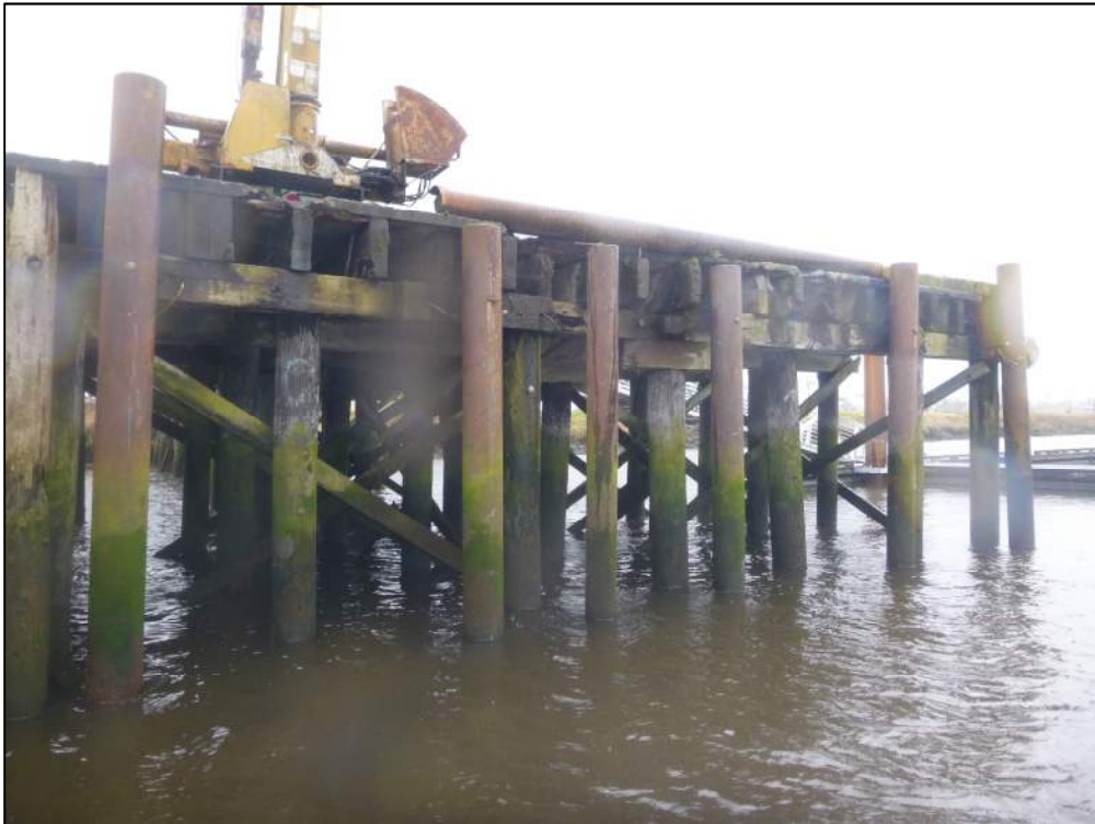
Photo 16. West Trestle Pile Cap Decay At Bent WT10
