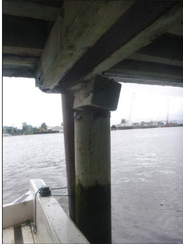
Photo 11. Displaced Pile At WP13/A
