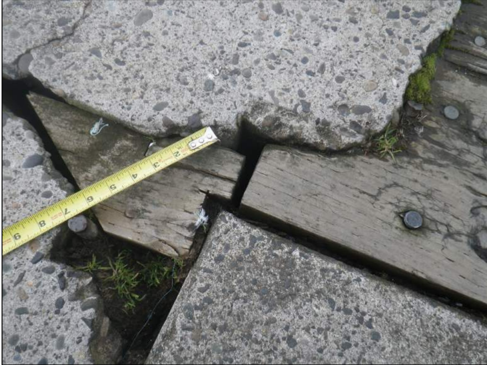
Photo 25. West Trestle Spall In Deck At WT8
