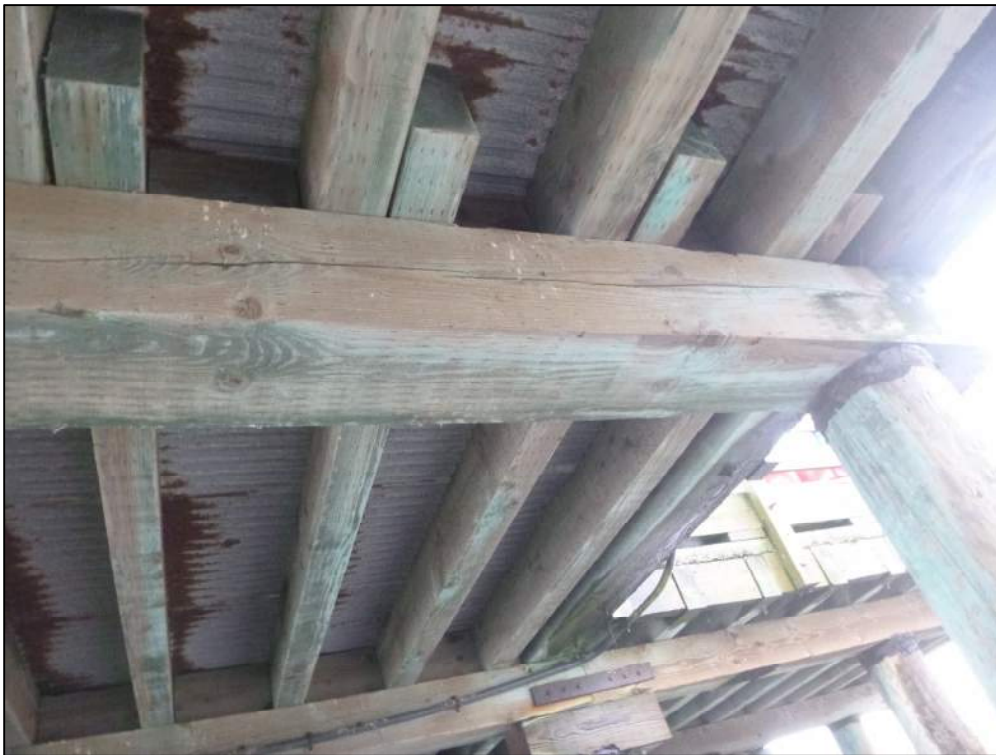
Photo 30. Work Pier Typical Deck Corrosion (Bent WP25)
