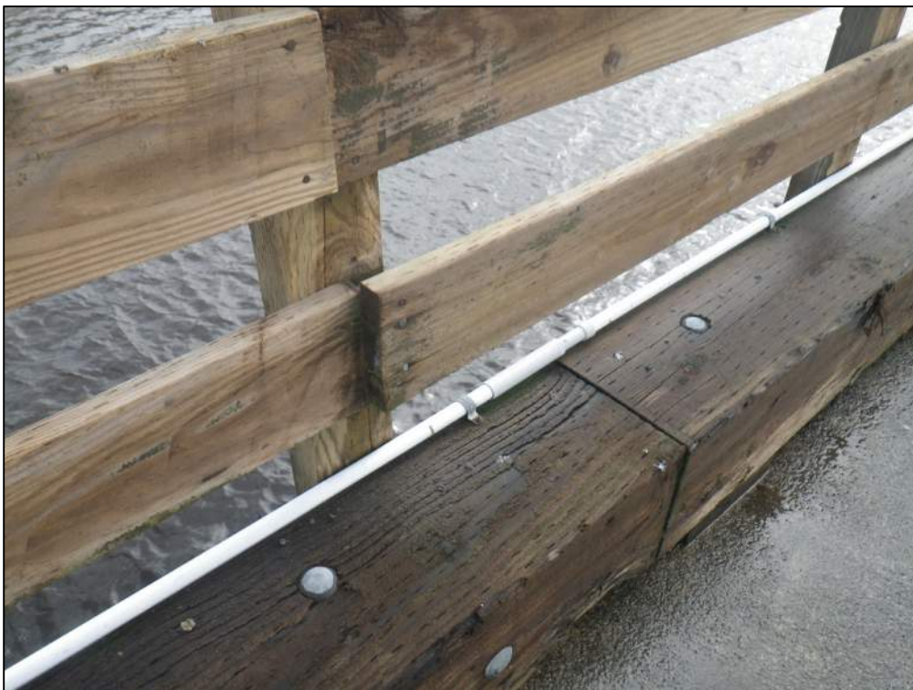
Photo 38. Work Pier Loose Connection At Horizontal Rail At WP28
