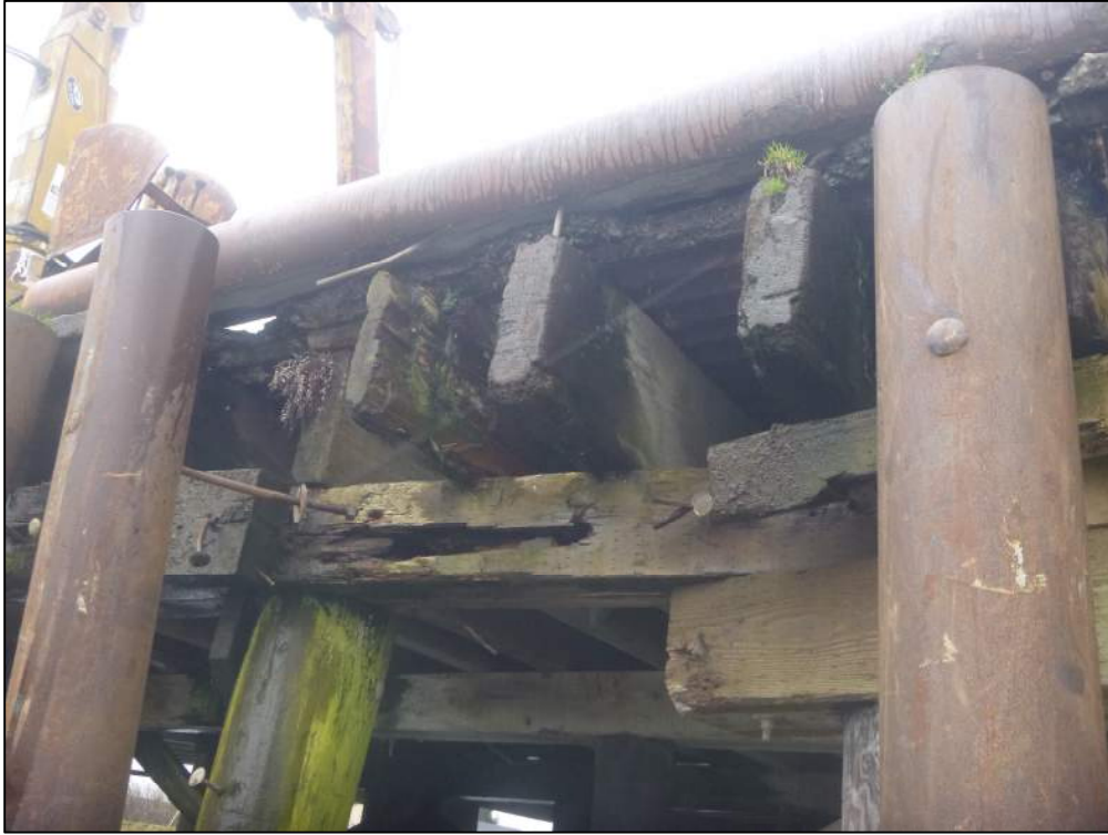
Photo 15. West Trestle Pile Cap Decay At Bent WT10
