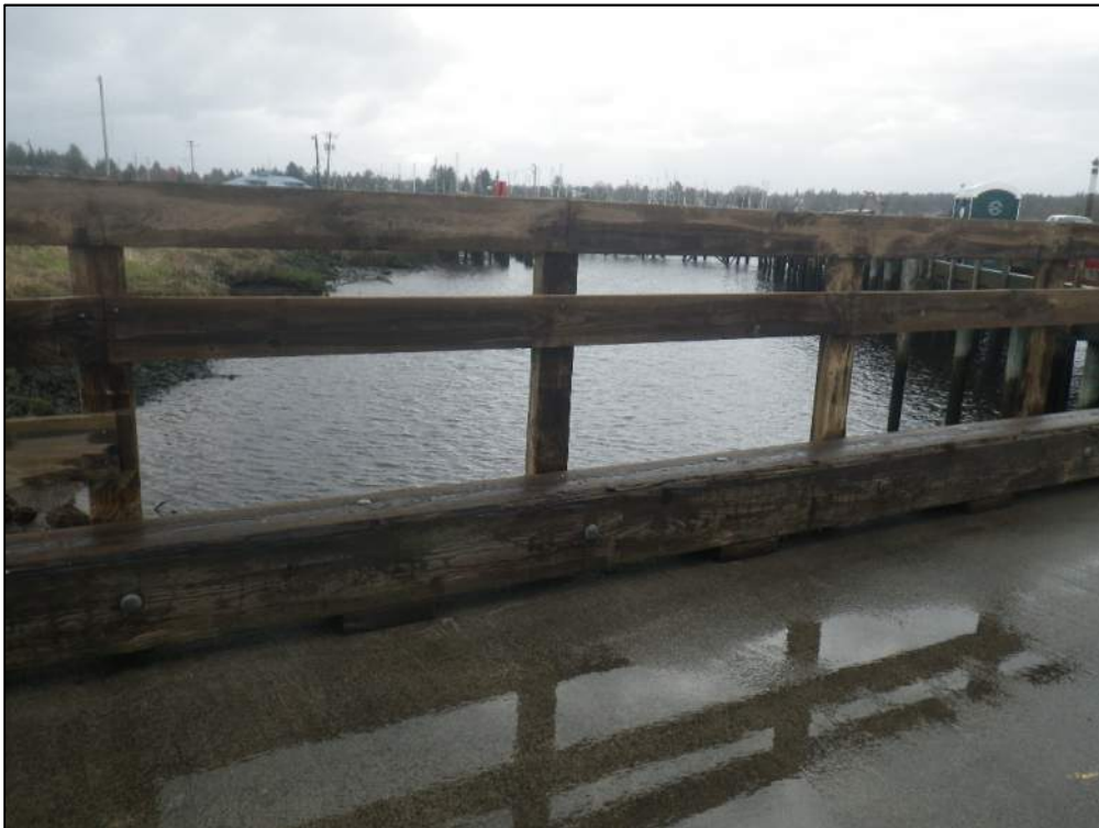
Photo 40. East Trestle Railing Missing Bottom Rail (Bent ET3 to ET6)
