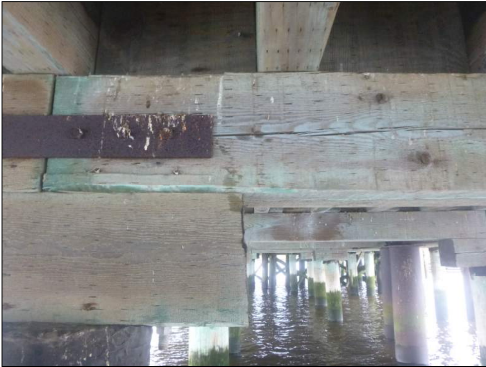
Photo 13. Typical Pile Cap Split (Bent WP10)
