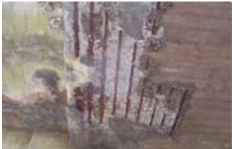
Condition State 5 (CS 5)
