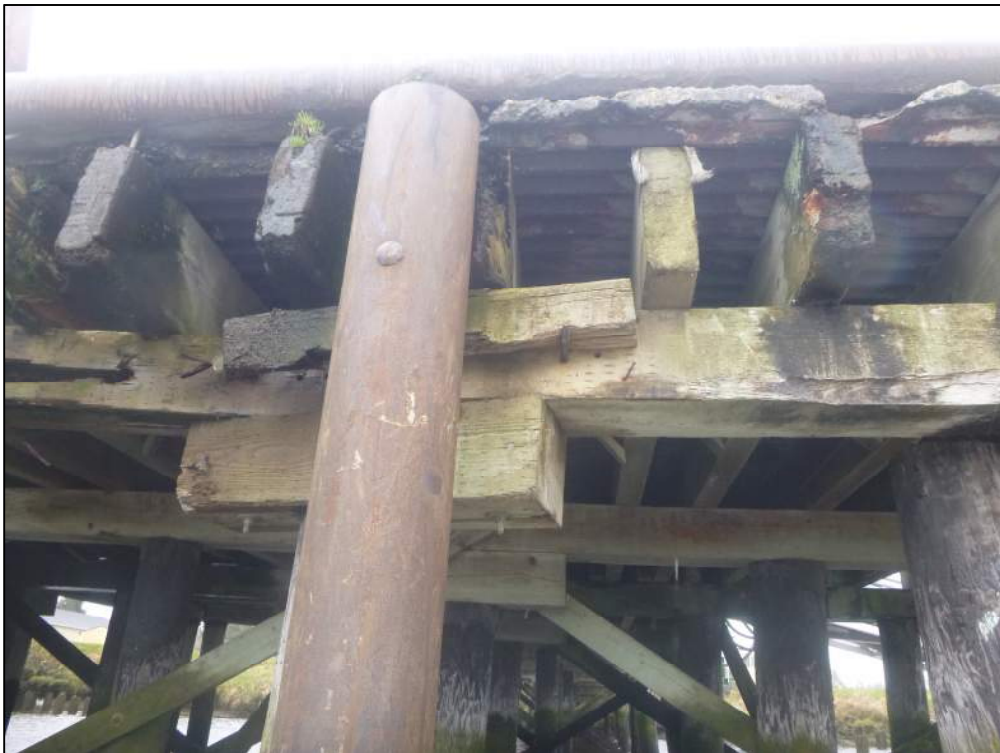
Photo 26. West Trestle Deck Edge Spalls And Metal Deck Corrosion At WT10
