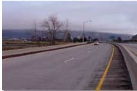
Condition State 1 (CS 1)
