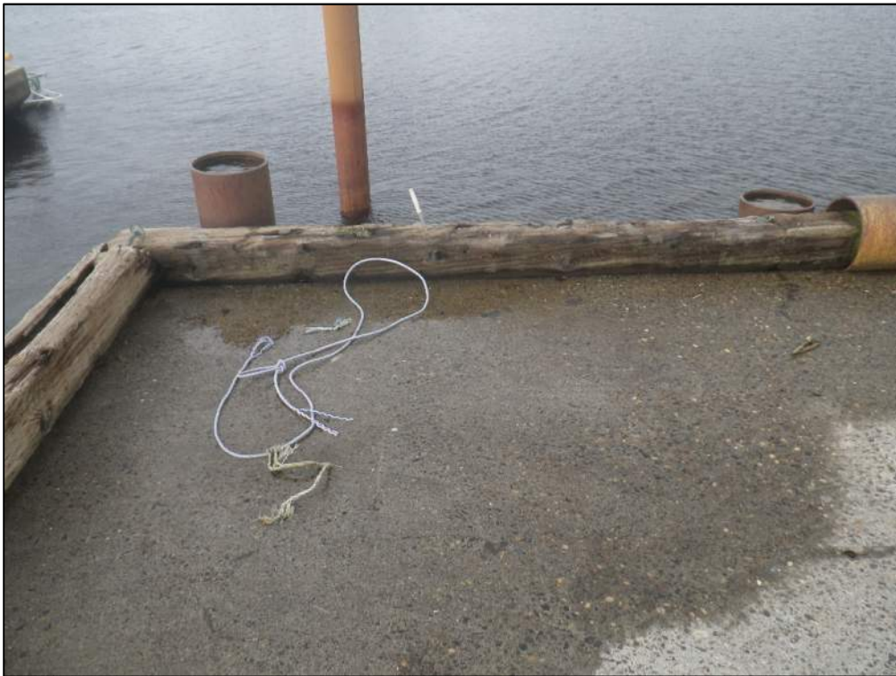
Photo 34. West Trestle Bullrail Deterioration At Bent WT10
