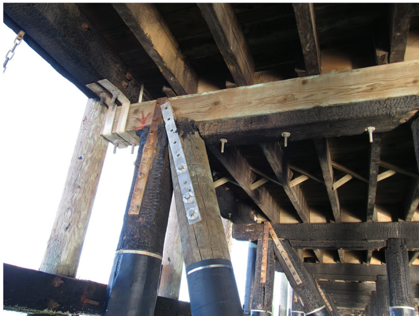
Fig. A-4. A view of the underside of a typical timber wharf. Note the stringers spanning between pile bents. Bridging is provided at midspan of the stringers to stabilize the members during installation. Source: Courtesy of Simpson Gumpertz & Heger, Inc., reproduced with permission.
