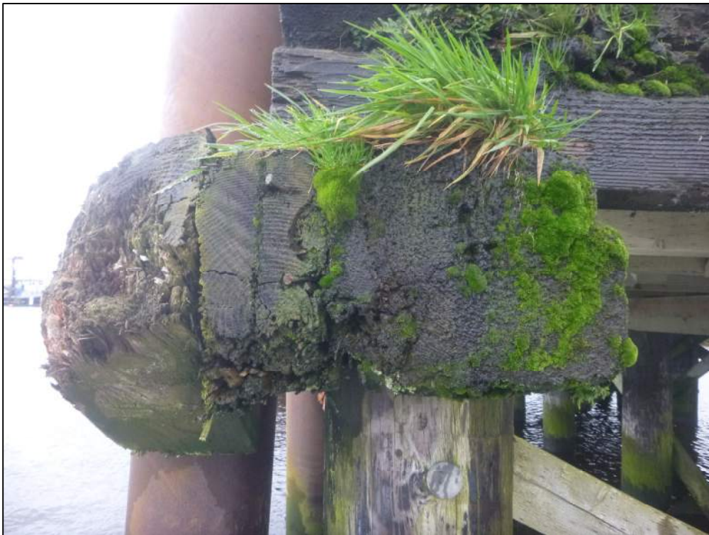
Photo 14. West Trestle Pile Cap Decay At Pile WT10/A
