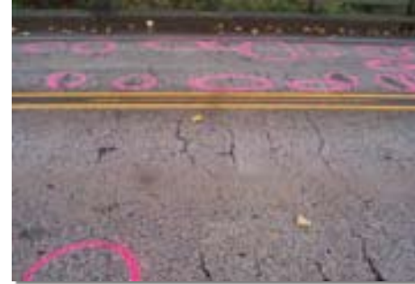
Condition State 4 (CS 4)
