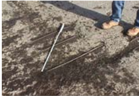
Condition State 3 (CS 3)
