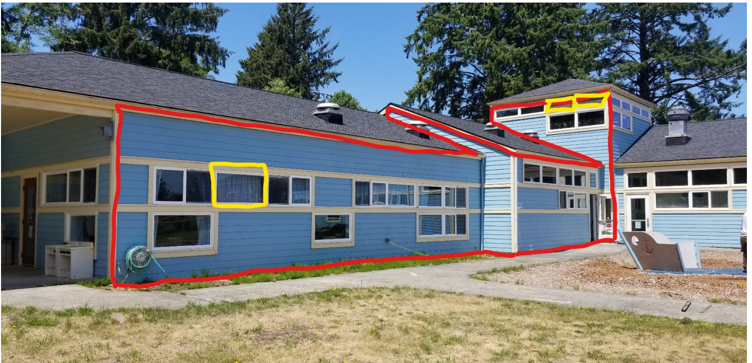
East Wall South Wing (Failed windows in yellow)
