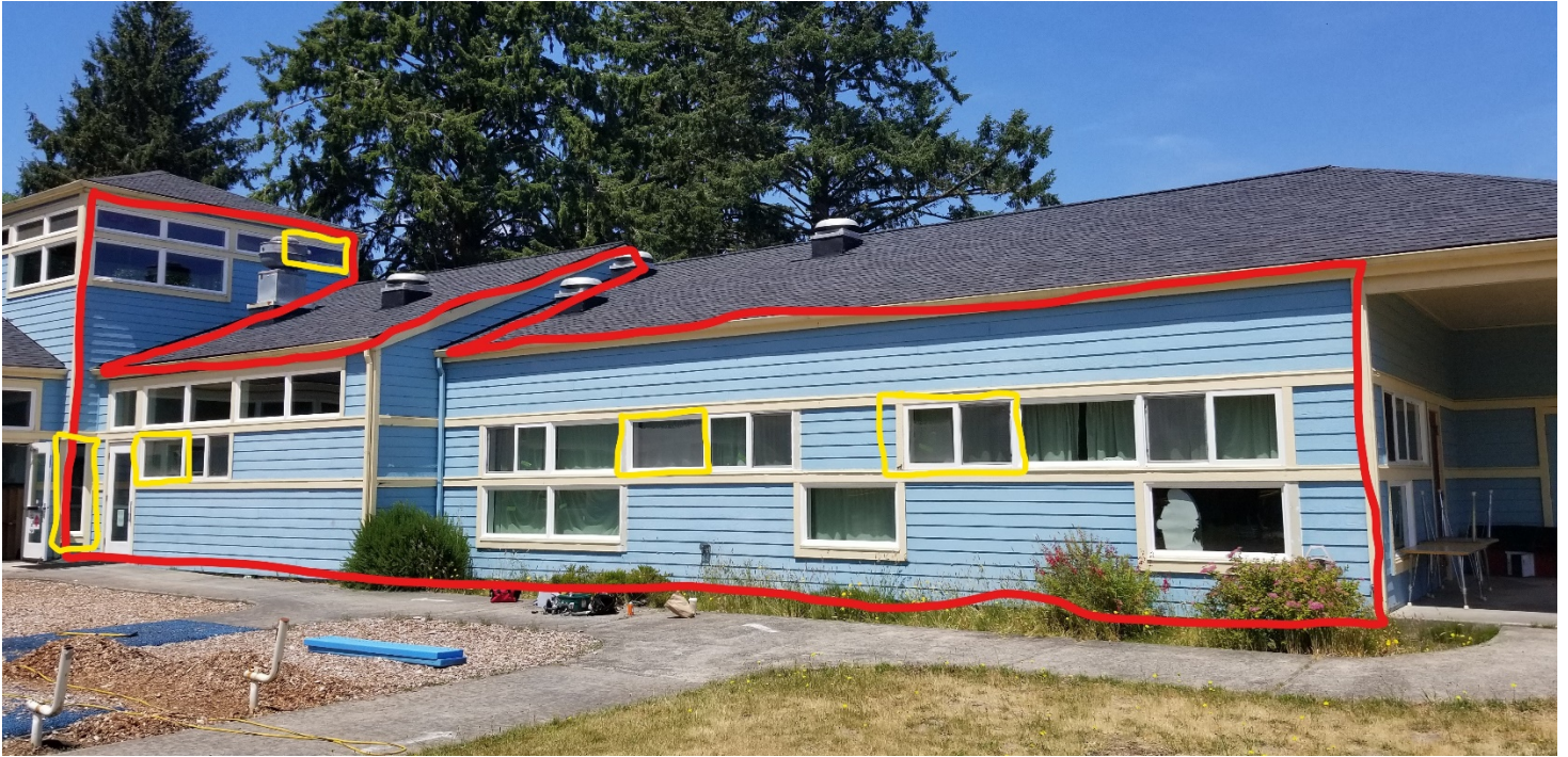
South Wall East Wing (Failed windows in yellow)
