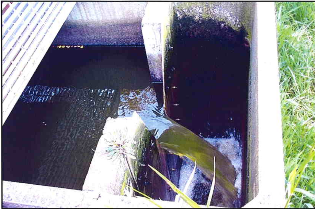
Figure 3: Effluent Discharge Control Weir
