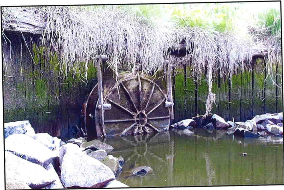
Figure 5: Tide Gate Beneath Levee
