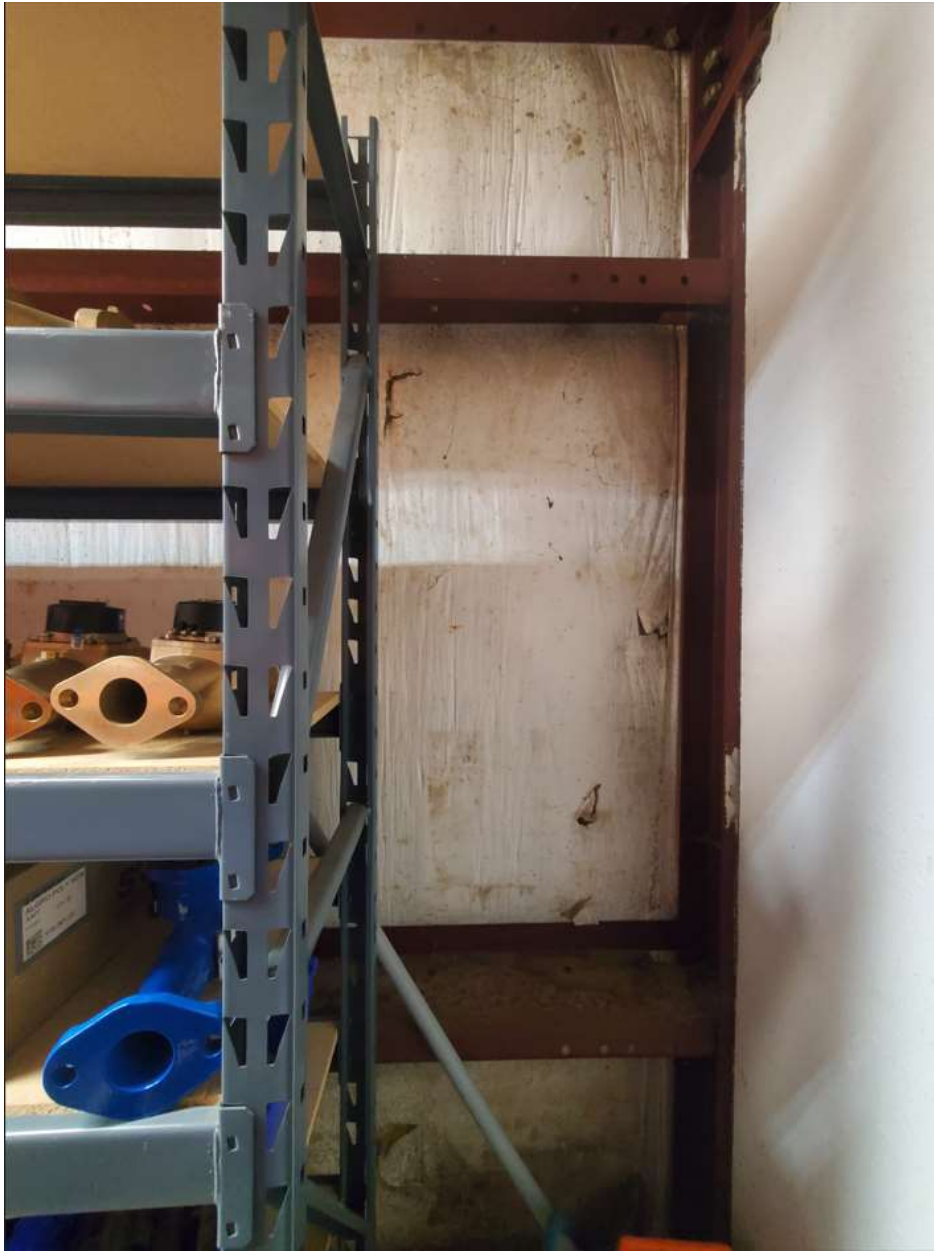
WALL INSULATION IN PARTS ROOM
