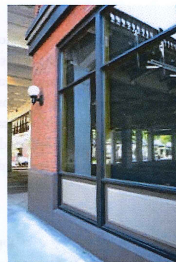
Contemporary storefront system example with aluminum-clad wood framed windows and integrated wood window base.
