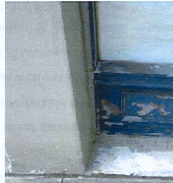
Base in need of paint
