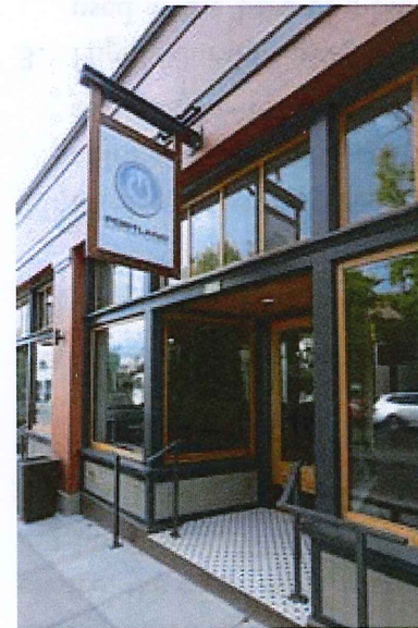
This recently updated storefront uses durable materials - wood + cement stucco. (SE 5th Ave and Clay St)
