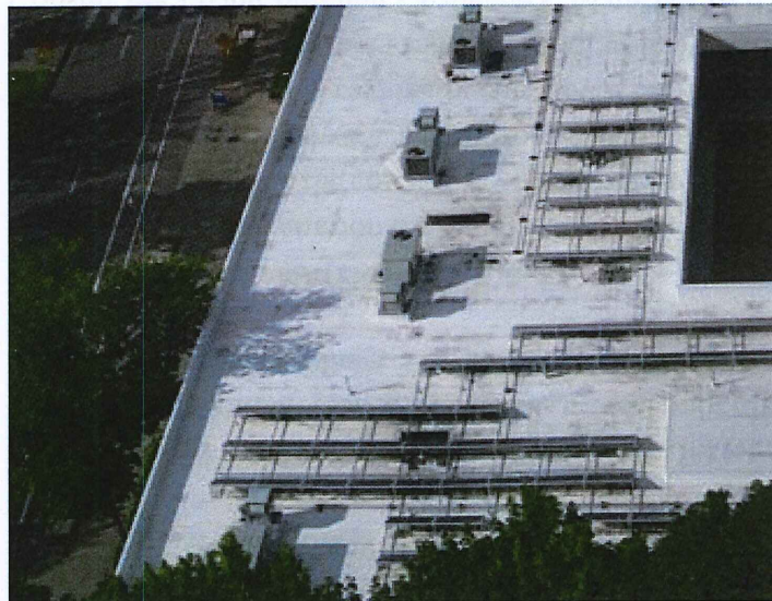
On site solar PV's are hidden from street view by this building's parapet (SW 1st Ave and Harrison St)
