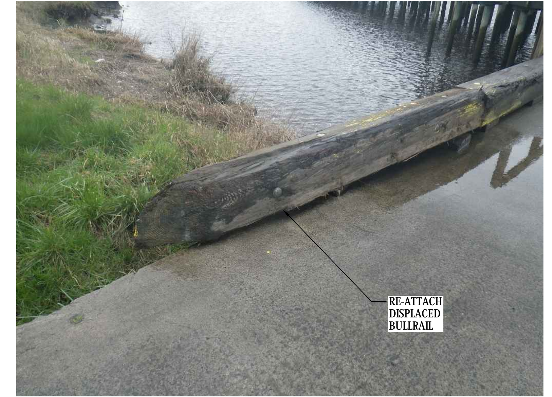
15 PHOTO - DISPLACED BULLRAIL AT ET0.5/B 5-12 SCALE: NTS
